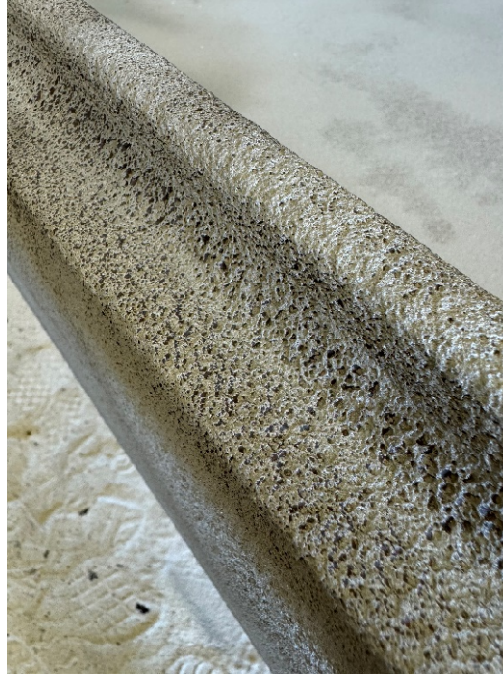
Photo 1 (Left): Hole in web of Beam D2
