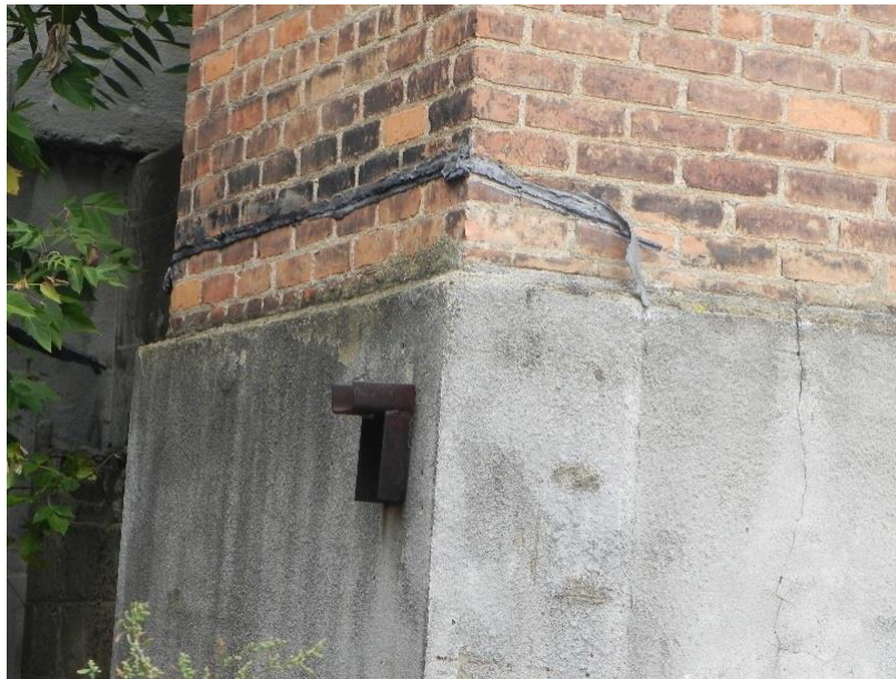
Photoset 3: Major horizontal cracks in brick above the concrete base along south and west sides.
