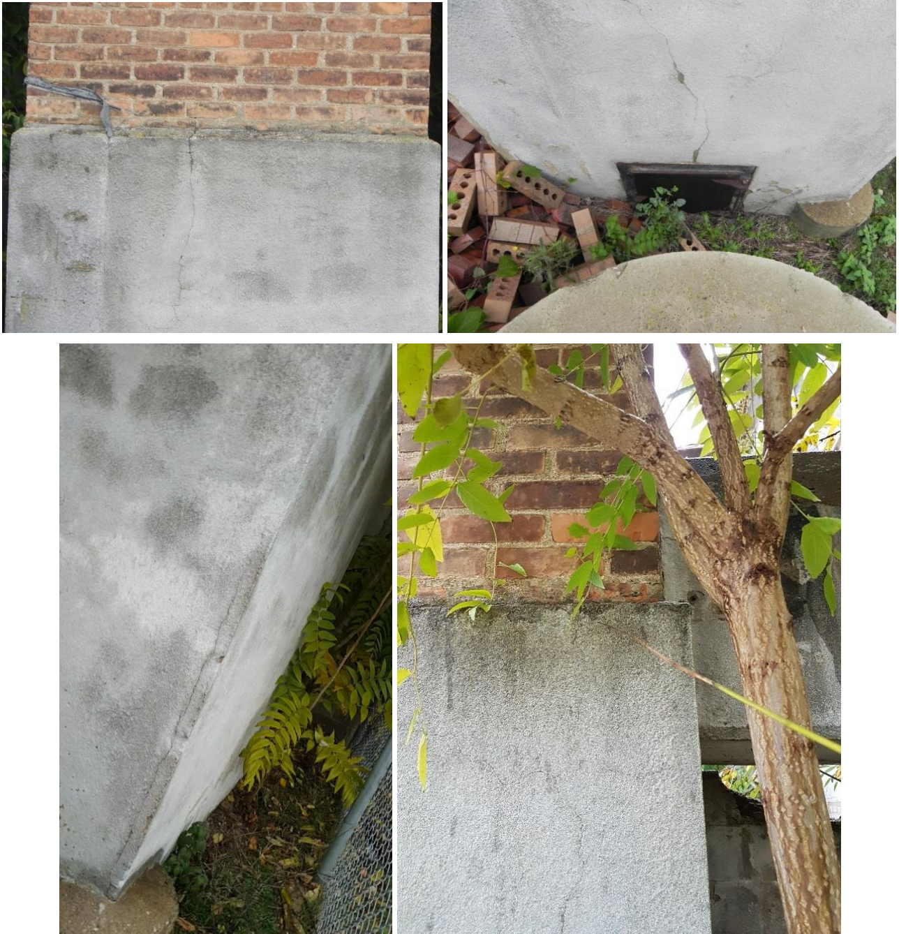
Photoset 2: Major vertical cracks along the south and east sides of the base.
