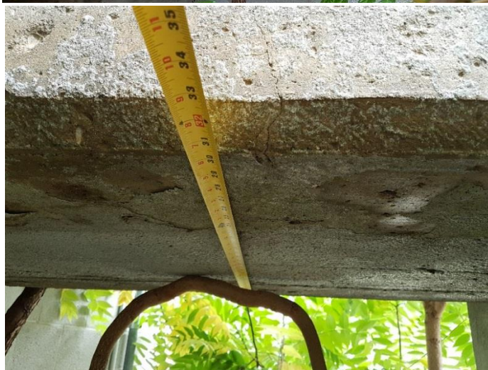
Photoset 4: Cracks in concrete beam and the adjacent building frame.
