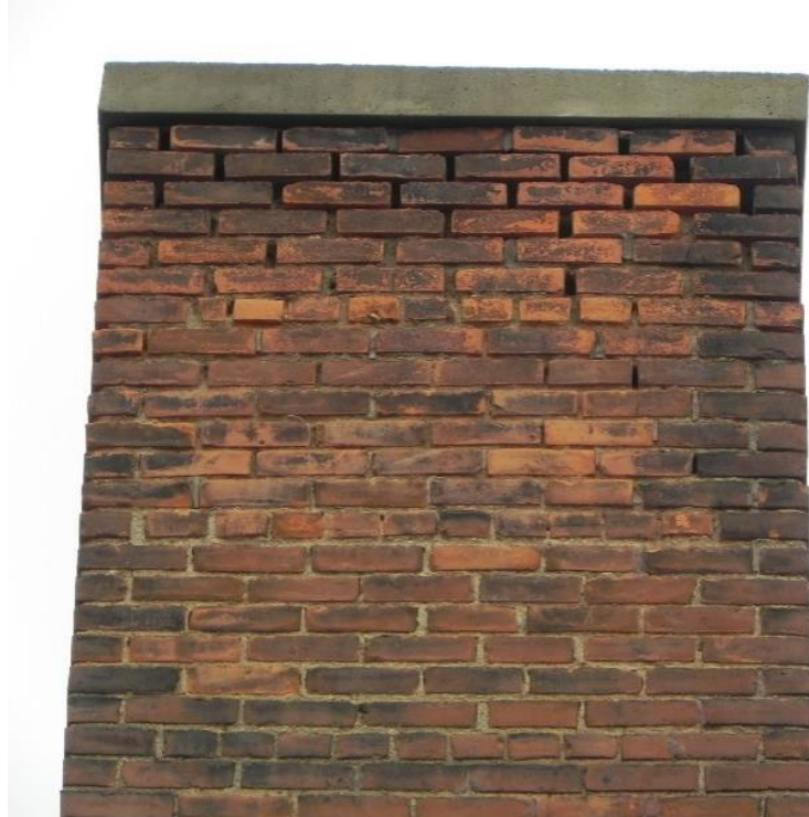
Photoset 1: Loose bricks and lack of mortar joints at top of chimney.
