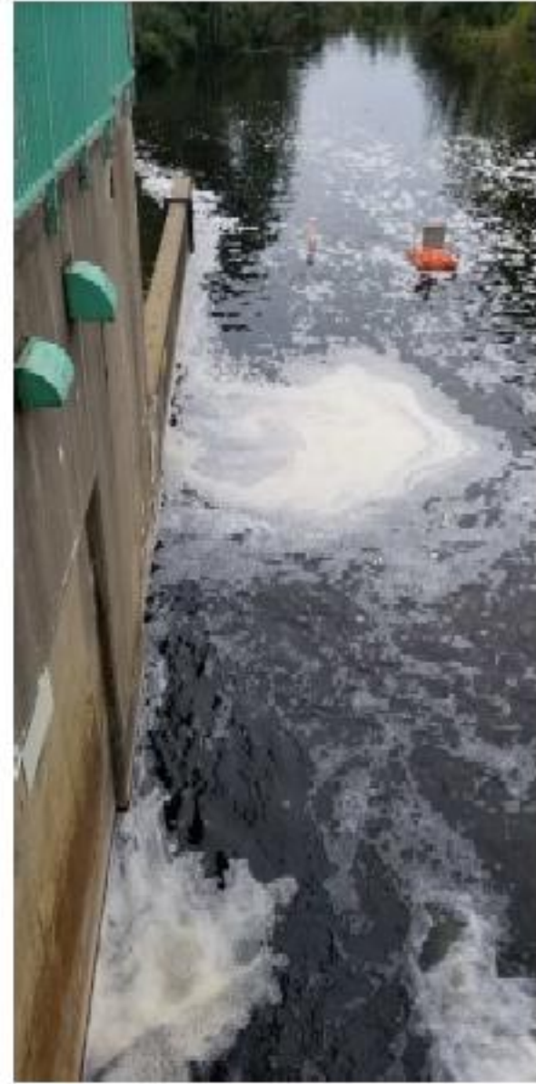
Foam at the Hubbell Pond Dam in Milford (9/8/2018)
