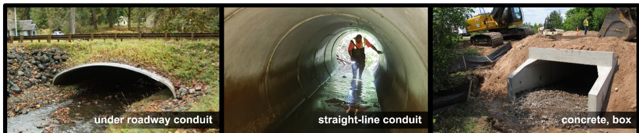
Figure C-2: Examples of culverts. Culverts allow water to pass under the roadway (left), they are straight-line conduits with no intermediate drainage structures (middle), and they come in various materials (left: metal; middle and right: concrete) and shapes (left: arch; middle: round; right: box).
