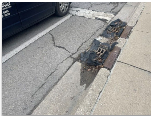
Drainage Grate Alignment on Ann Street
