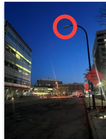
Non-working Light Fixture at Ann Street and Zina Pitcher Place
