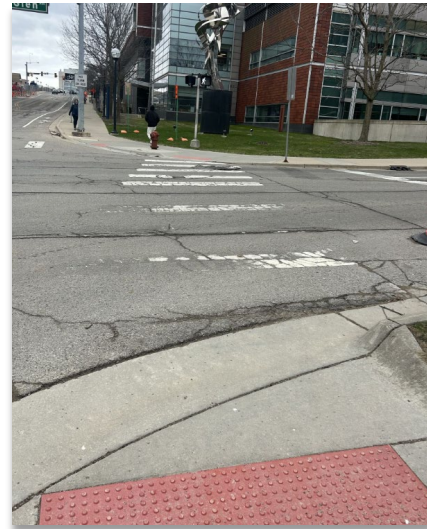
Faded Crosswalk Markings
