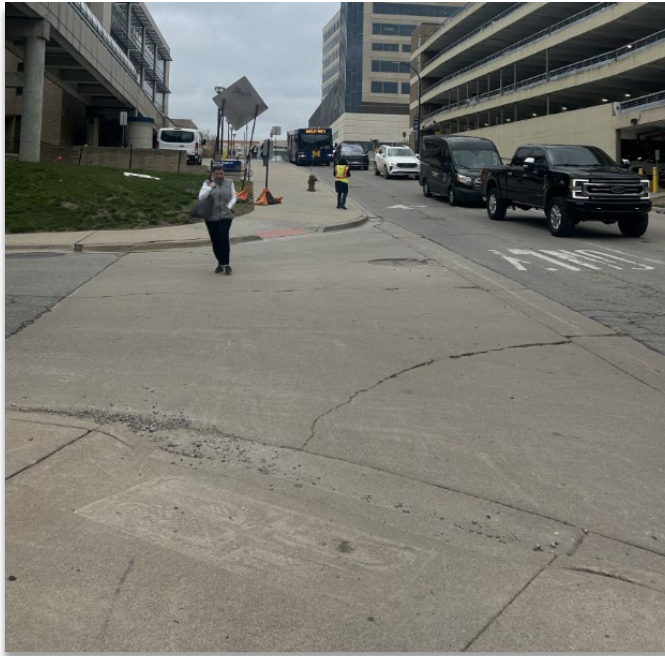
Missing Pavement Marking
