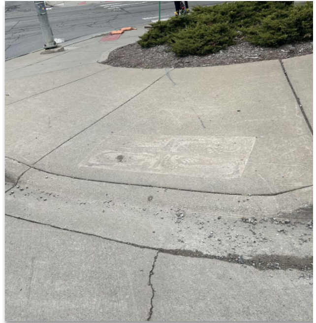
Missing Detectable Warning Pad
