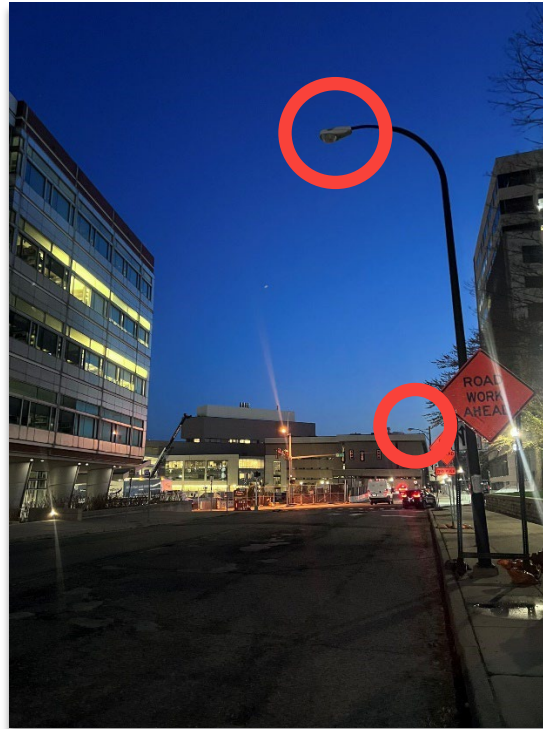
Figure 36 - Non-functional light fixtures at Ann Street and Zina Pitcher Place
