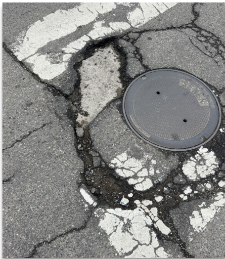
Broken Pavement in the Crosswalk
