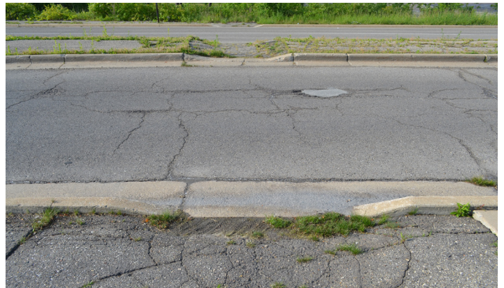
Sidewalks and pedestrian crosswalks are deteriorated
