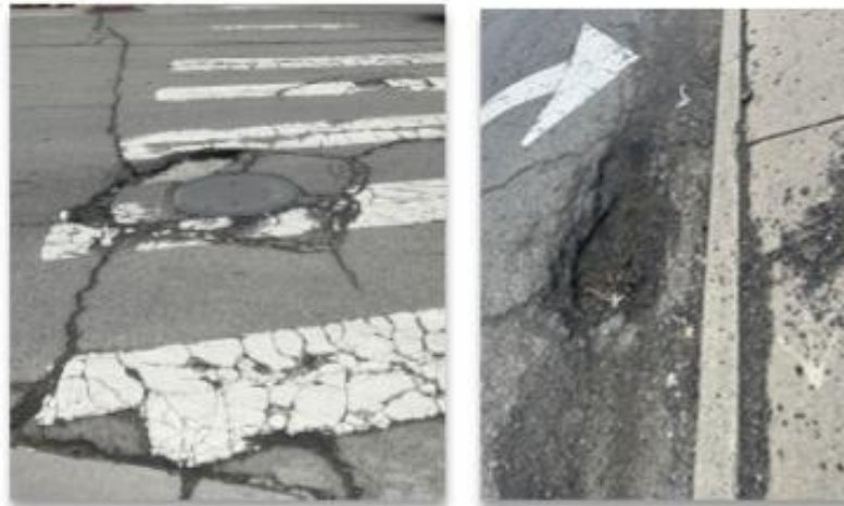
Cracked Pavement Throughout the Study Area
