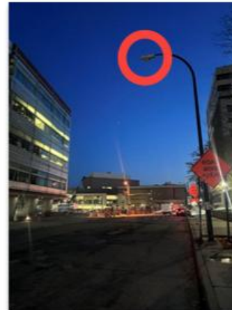
Non-working Light Fixture at Ann Street and Zina Pitcher Place
