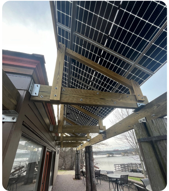
Solar array installed at Gallup Park.
