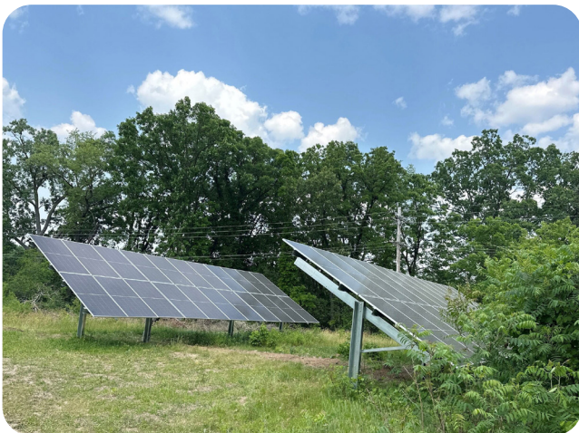
Solar array installed at Huron Hills Golf Course.
