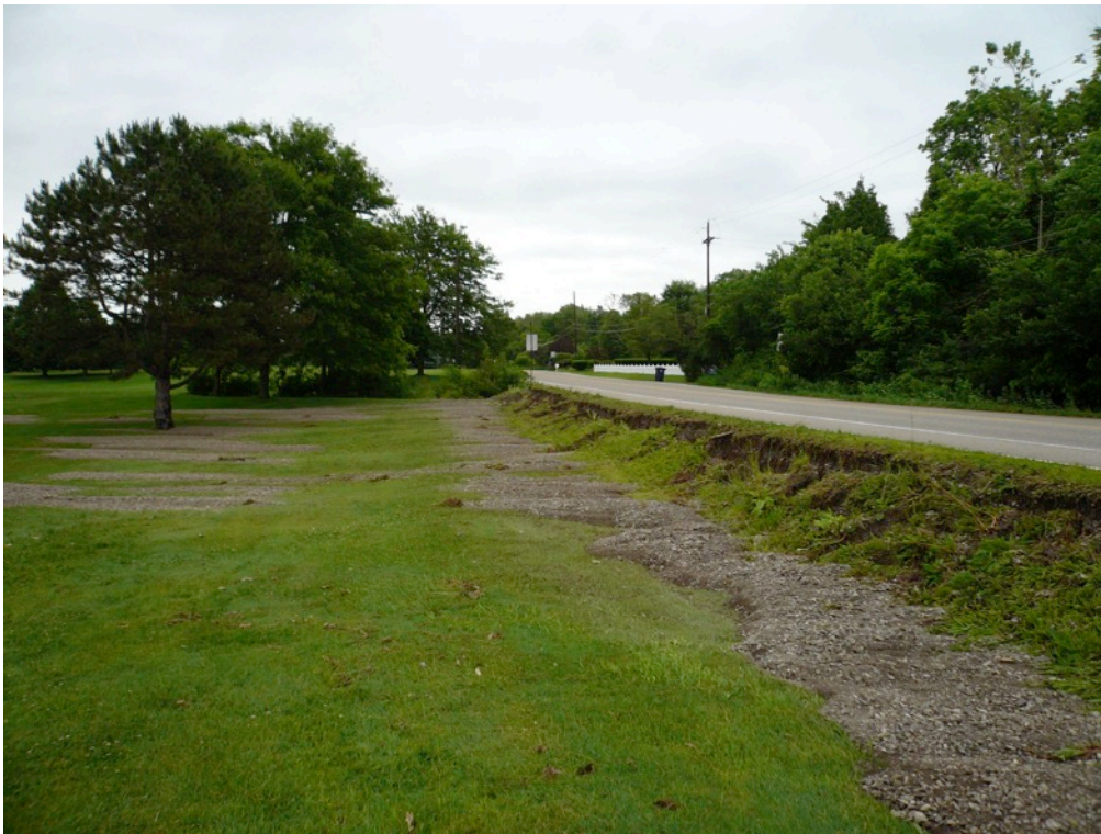
A. Erosion of embankment following rainstorm. Next to E Huron River Dr. just east of Elmwood by Huron Hills Golf course, (same area as first picture) (~June 6, 2010) (Water from another storm overflowed E Huron River Dr ~July 26, 2011)
