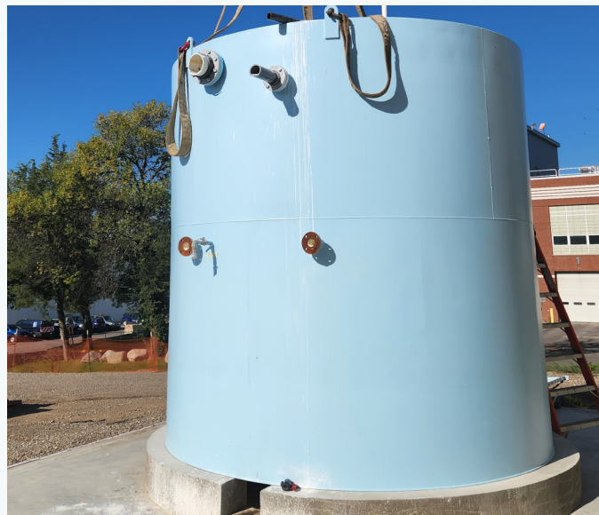
Pre-treatment tank (clarifier) for pilot testing
