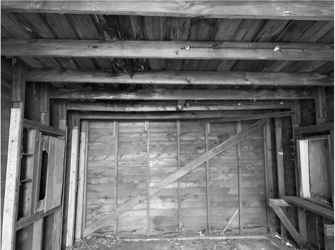
PHOTO #9 – DISCONTINUOUS STUDS
