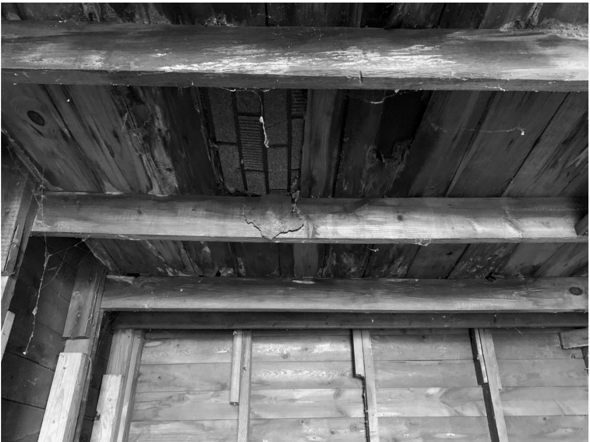
PHOTO #10 – DETERIORATED JOISTS/DECKING
