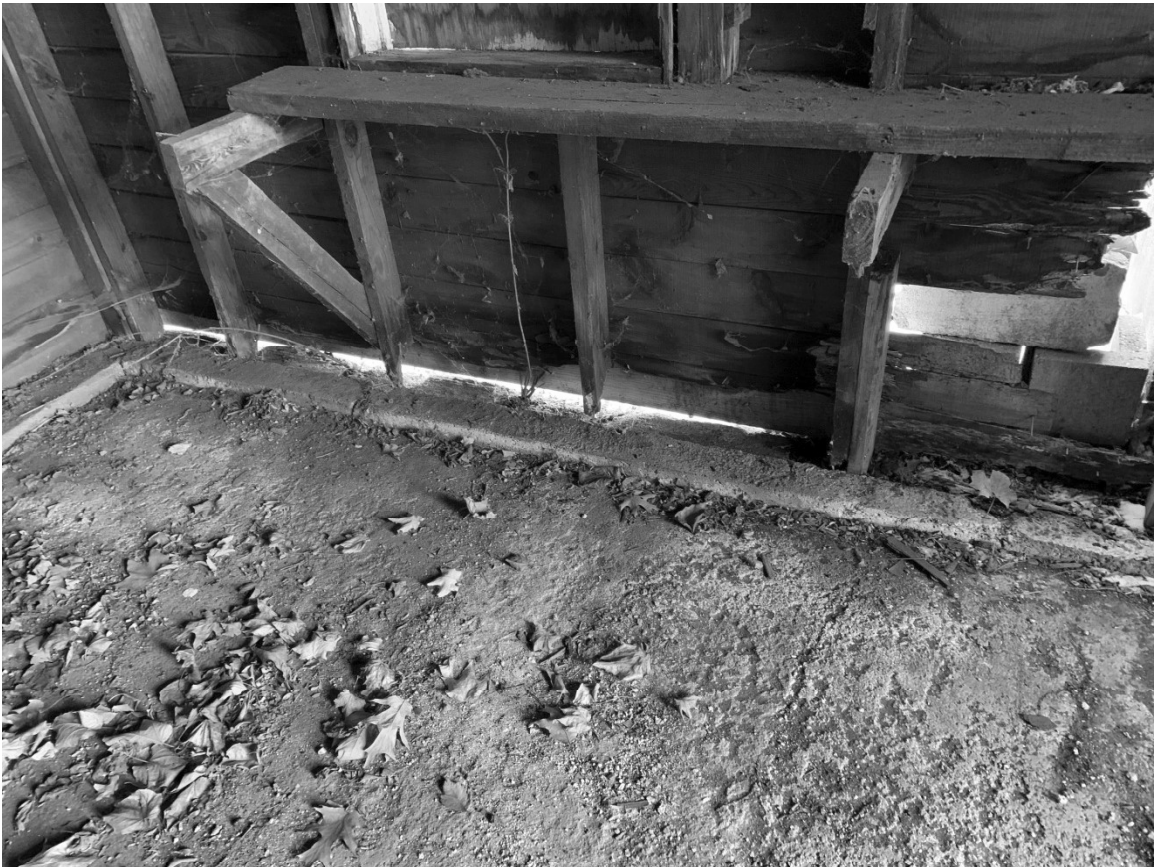
PHOTO #5 – ROTTED STUDS @ BASE
