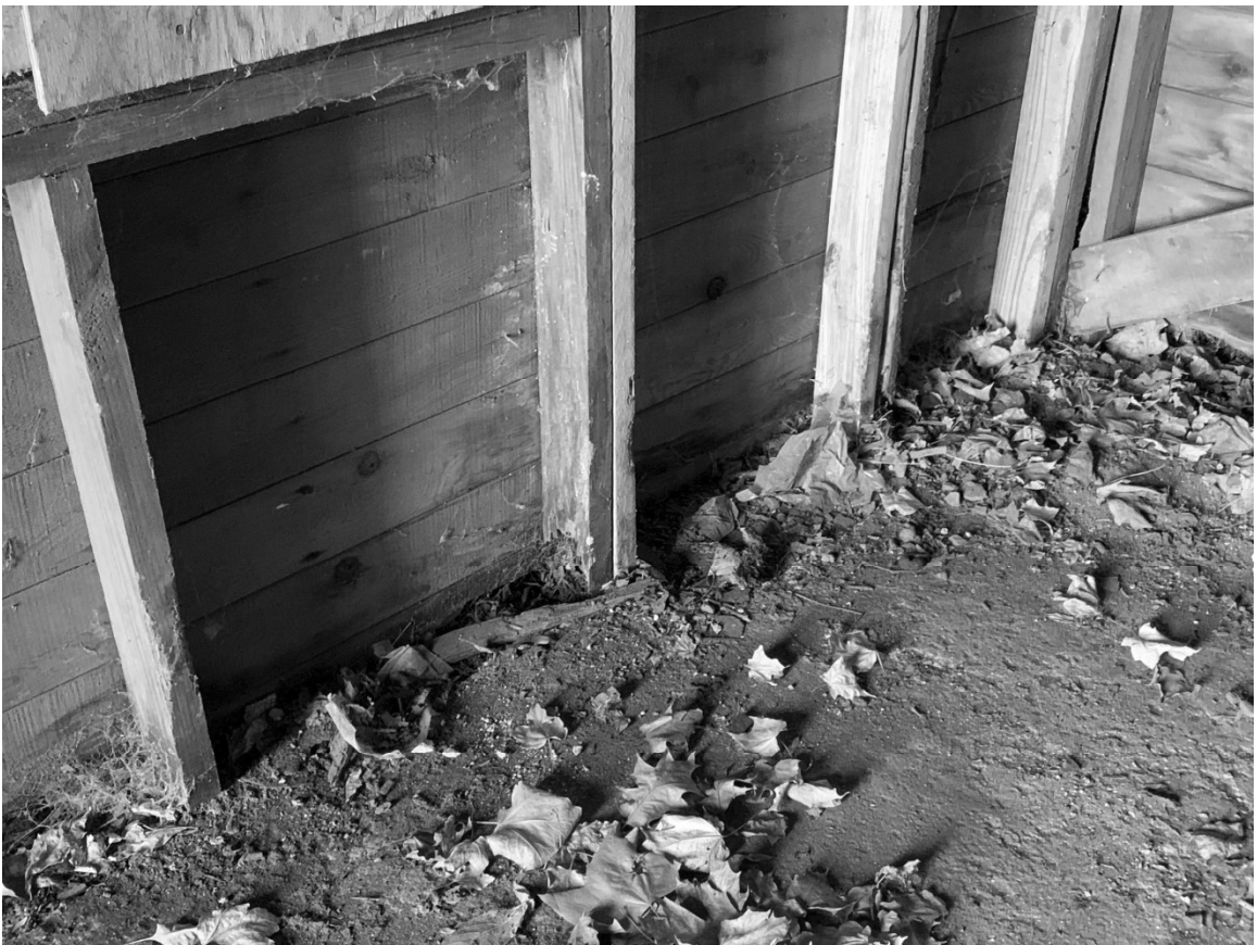
PHOTO #6 – ROTTED STUDS @ BASE
