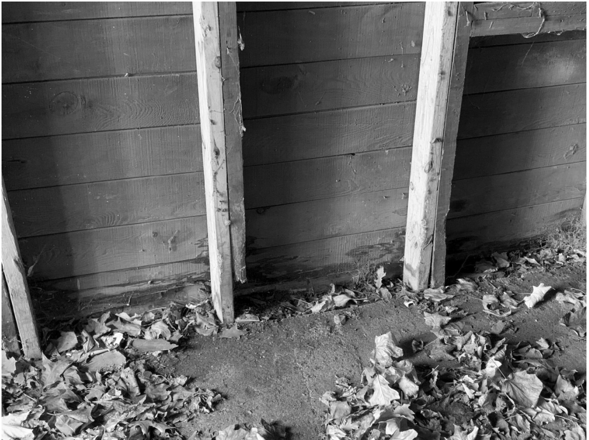
PHOTO #7 – ROTTED STUDS @ BASE
