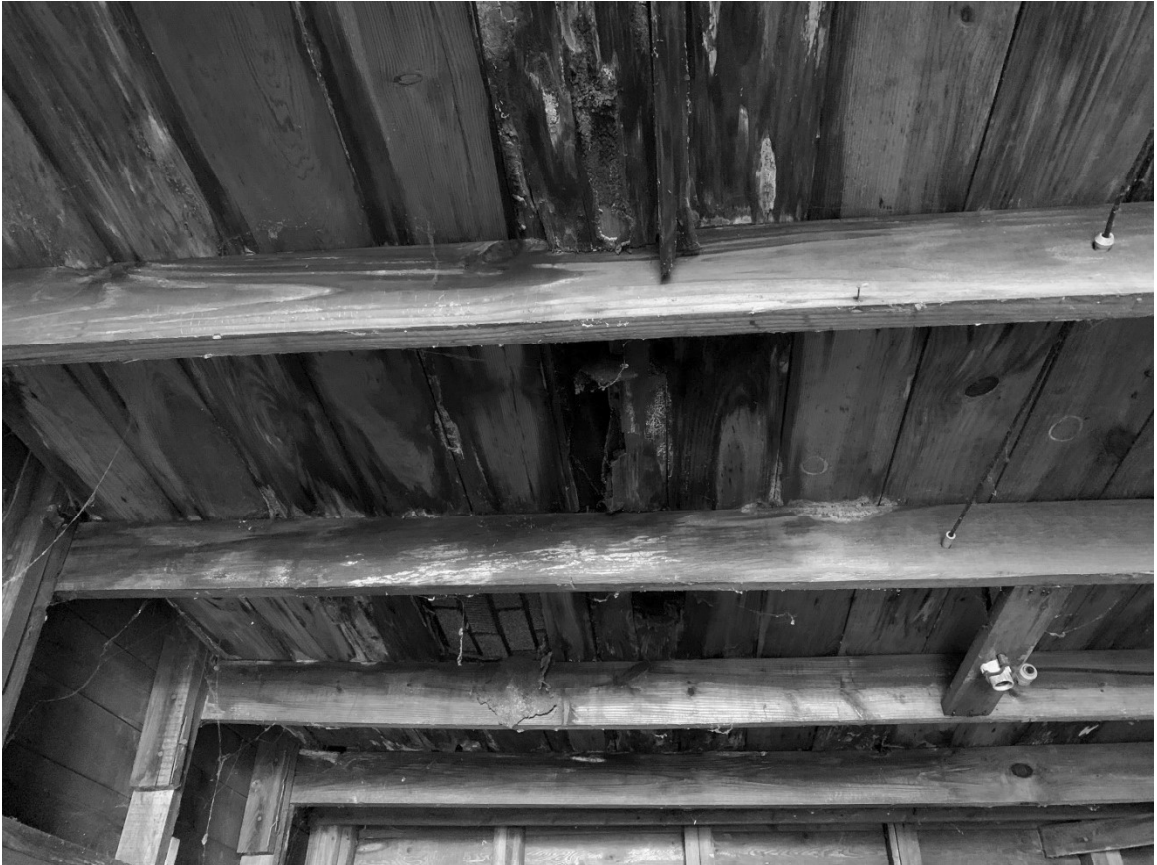
PHOTO #11 – DETERIORATED JOISTS/DECKING
