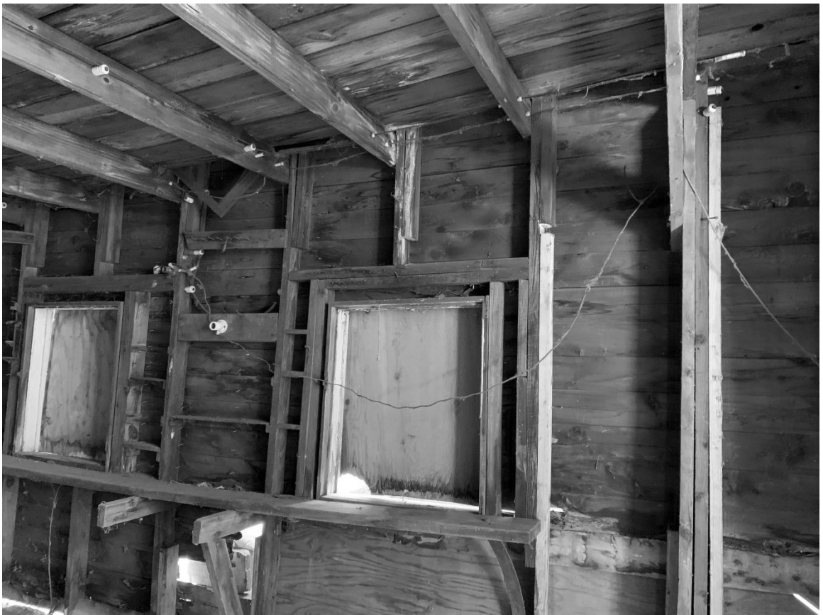
PHOTO #8 – DISCONTINUOUS STUDS
