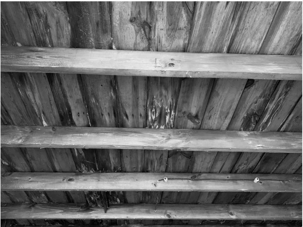
PHOTO #12 – DETERIORATED JOISTS/DECKING
