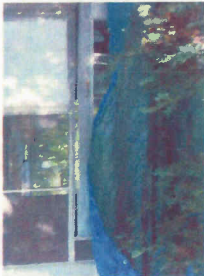
Sun Room and Roof Tarp
