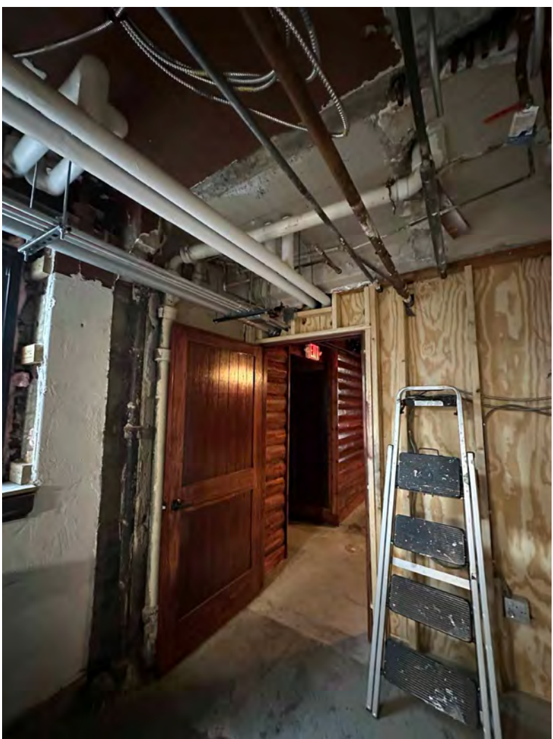
6 VIEW 6 A5.1 View of newly installed HVAC piping and conduit along with existing structure and recent wall renovations
