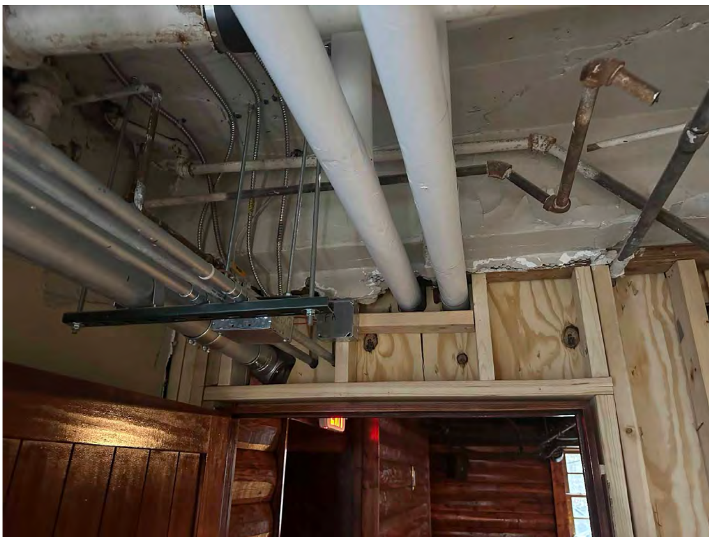
8 VIEW 8 A5.1 View of newly installed HVAC piping and conduit along with existing structure and recent wall renovations
