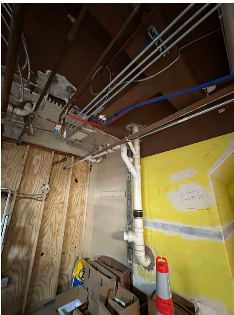
7 VIEW 7 A5.1 View of newly installed HVAC piping and conduit along with existing structure and recent wall renovations
