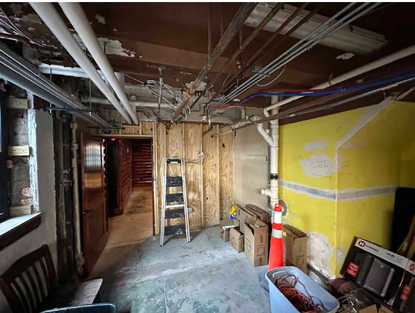
5 VIEW 5 A5.1 View of newly installed HVAC piping and conduit along with existing structure and recent wall renovations
