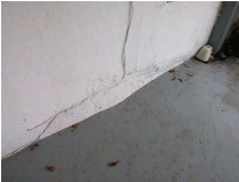
Figure 2. Bulging of exterior stucco finish along adjacent wall to east wall of home.
