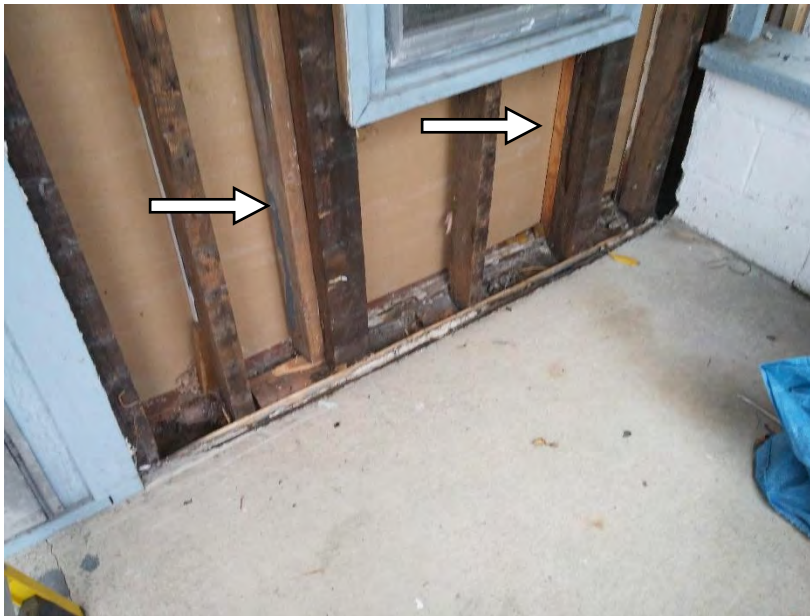
Figure 4. Newer wood 2x furring members added to original wall framing.
