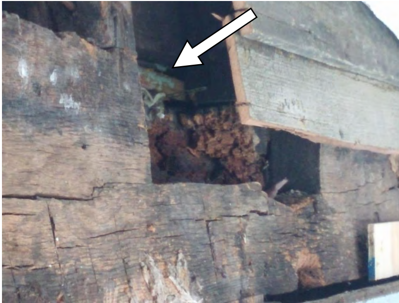
Figure 7. Decay of second floor perimeter timber beam. Arrow pointing to edge of second floor decking.
