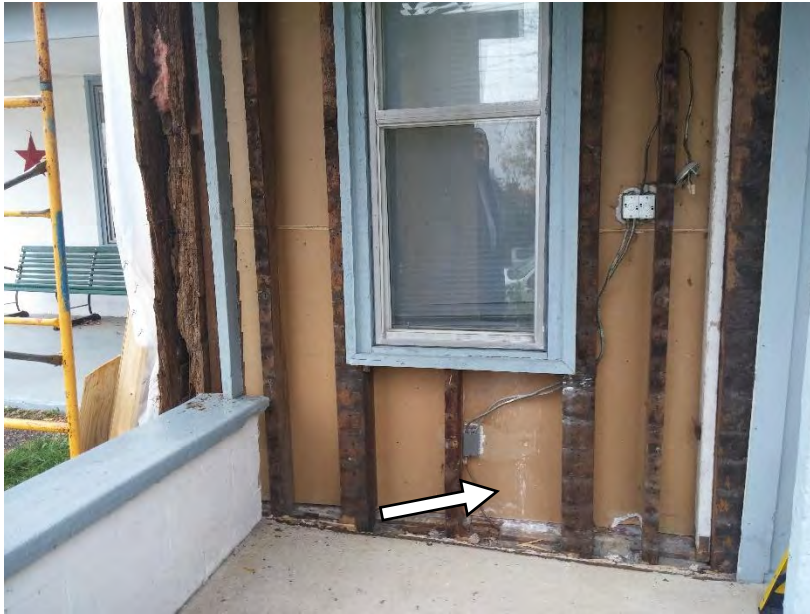
Figure 1. Exterior cladding removed in 2016 exposing wood framing of east wall of home. Arrow is pointing to water staining on the backside of the gypsum board interior finish.
