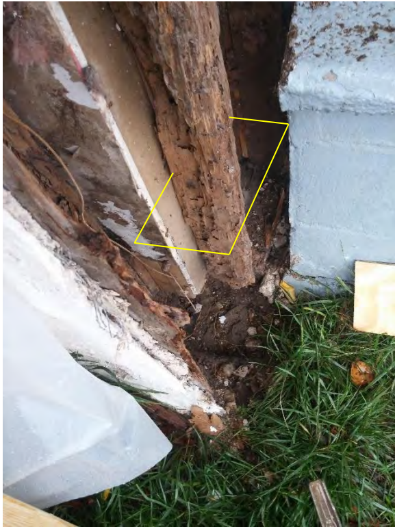
Figure 5. Decayed timber corner column; yellow lines indicate approximate original section size.
