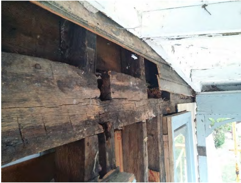
Figure 3. Rotated second floor timber beam. Note 2x ledger for porch roof rafters secured to east wall timber framing.
