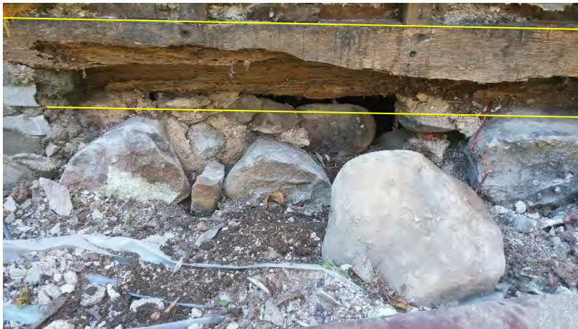
Figure 6. Loose stone and missing mortar of stone foundation. Decayed summer beam atop stone foundation. Yellow lines indicate approximate original section depth.
