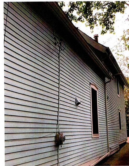
SOUTH ELEVATION (LOOKING EAST): NEW WINDOWS AT REAR OF HOUSE, NEW TEMPERED WINDOW IN ENTRY TO MATCH EXISTING KITCHEN WINDOW
