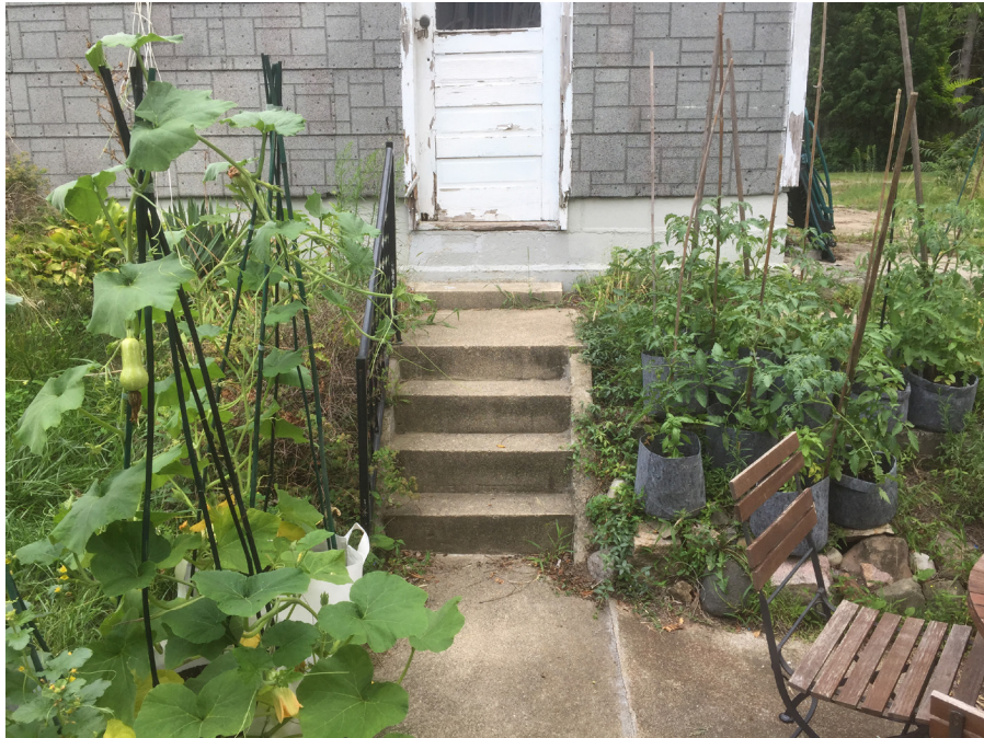
Existing steps from back of house to upper level garage, cinder block retaining walls buried behind vegetation.
