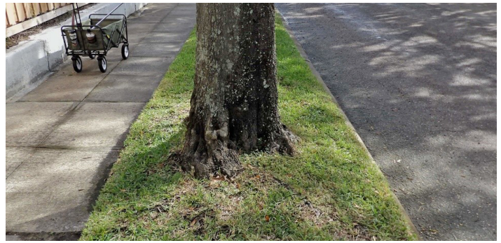
Figure 3. A large laurel oak ( Quercus laurifolia ) planted in a narrow planting strip. The lighter-colored pavement squares on the left were most likely replacements due to tree root damage. Credits: Deborah R. Hilbert, UF/IFAS
