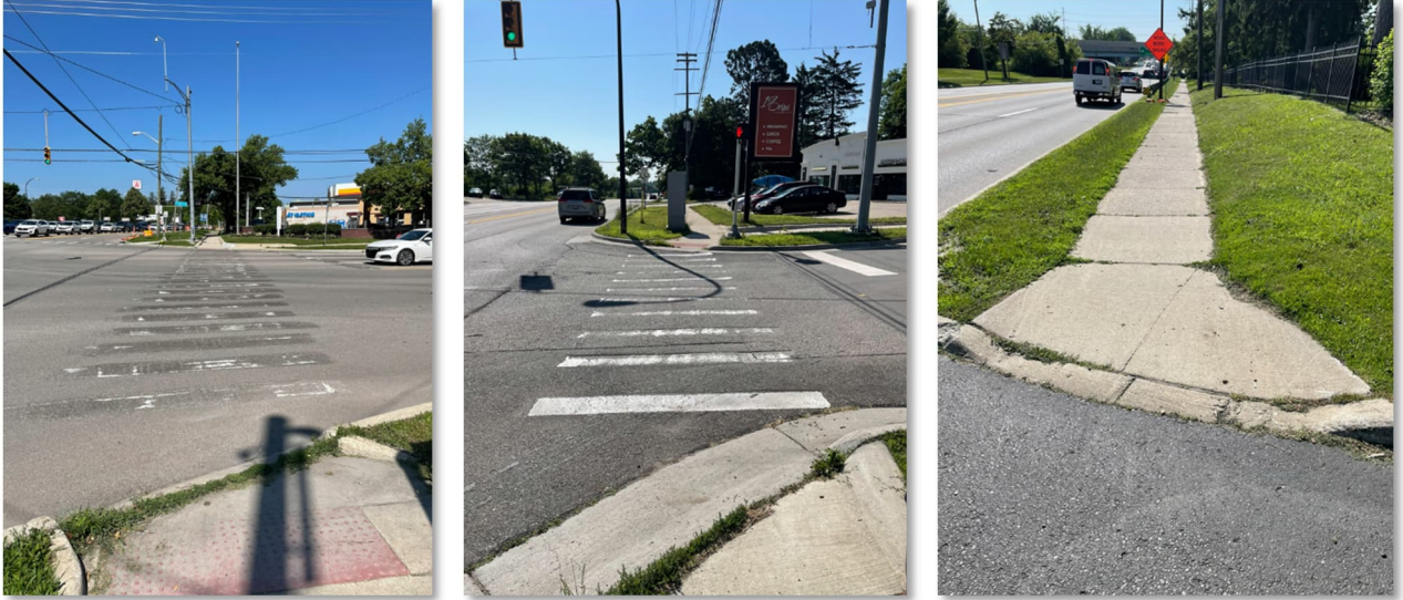
Figure 16 – Non-ADA Compliant Ramps and Faded Pavement Markings
