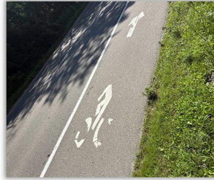
Worn Bike Lane Pavement Marking
