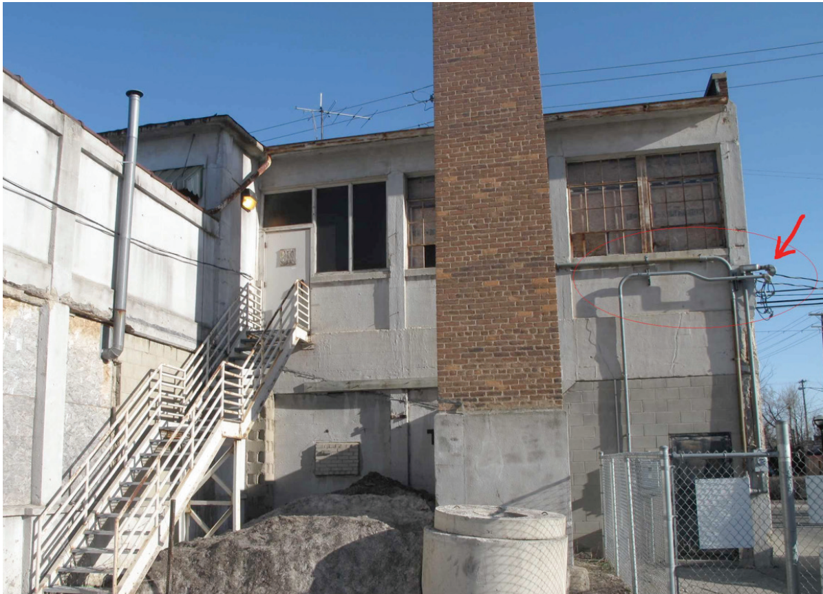
Picture E1: Existing electrical service at corner of buildings A & B
