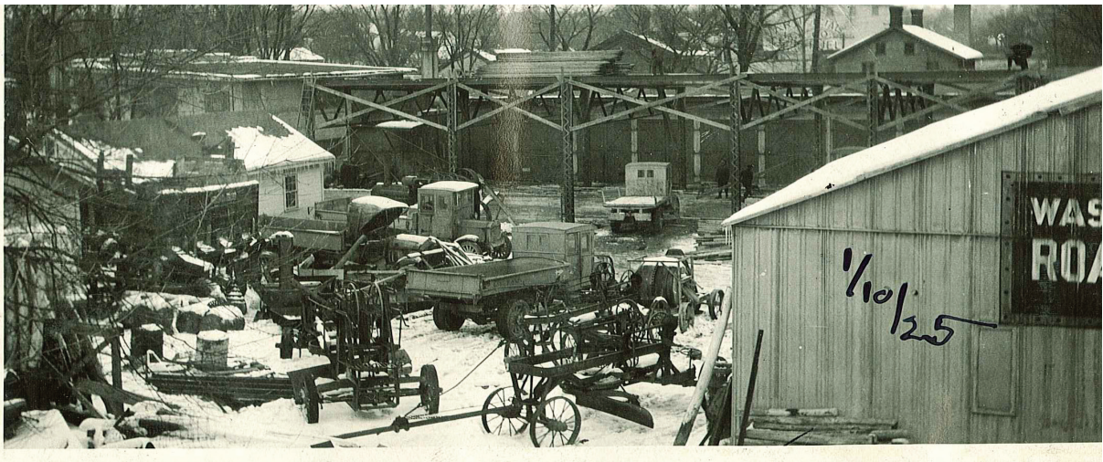
January 10, 1925 photo of the new Warren trusses on the garage going up in front of the old 12 bay garage. The existing concrete machine shop is visible on the left. As the new garage was being erected, most of the old garage with the exception of the one story wall fronting Washington Street was demolished and a new second story was added.
