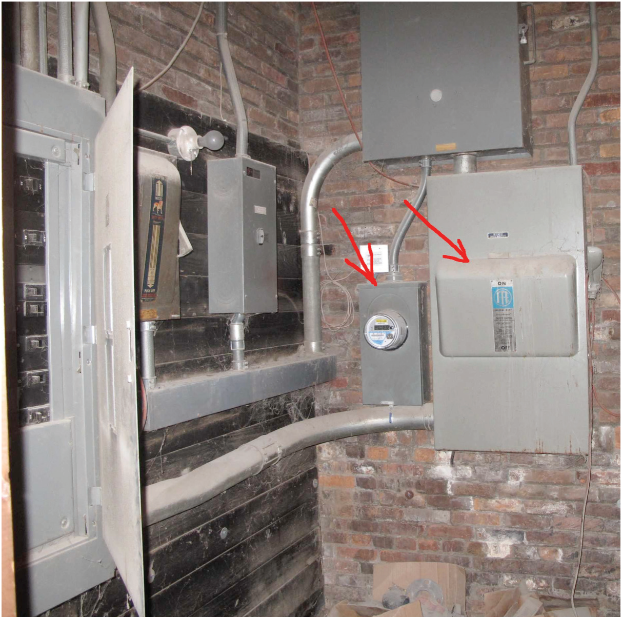
Picture E2: Existing electrical service at building D
