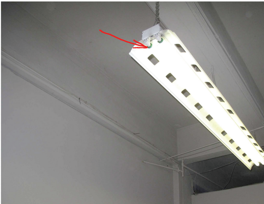
Picture E3: Existing lighting
