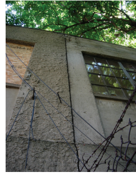
Photo with 1925 building (on left) and 1928 addition (on right). Stucco covers the earlier building, while the later addition was left uncovered.
