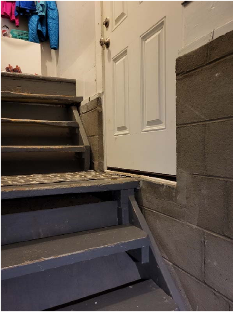
Interior basement stair – door overhangs landing and steps
