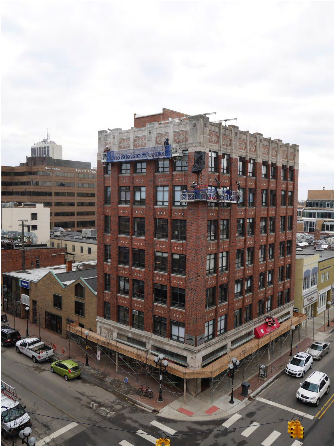
Photo taken by the applicant on March 20, 2014. The brick piers and mullions of the upper stories do not align with the storefront masonry below, and storefront window muntins also do not align with the brick masonry above. Scaffolding obscures a clear view of the storefronts and kickplates.
