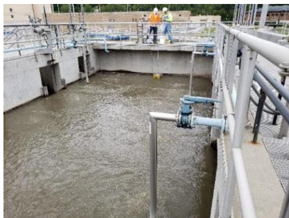
Figure 9: Flow Splitter Channels on the West Plant near the Screenings and Grit Building
