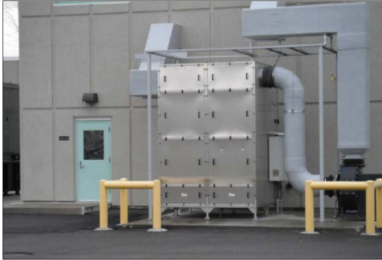
Figure 5-5. Photograph of a NEUTRALOX® Photoionization Unit Installation
