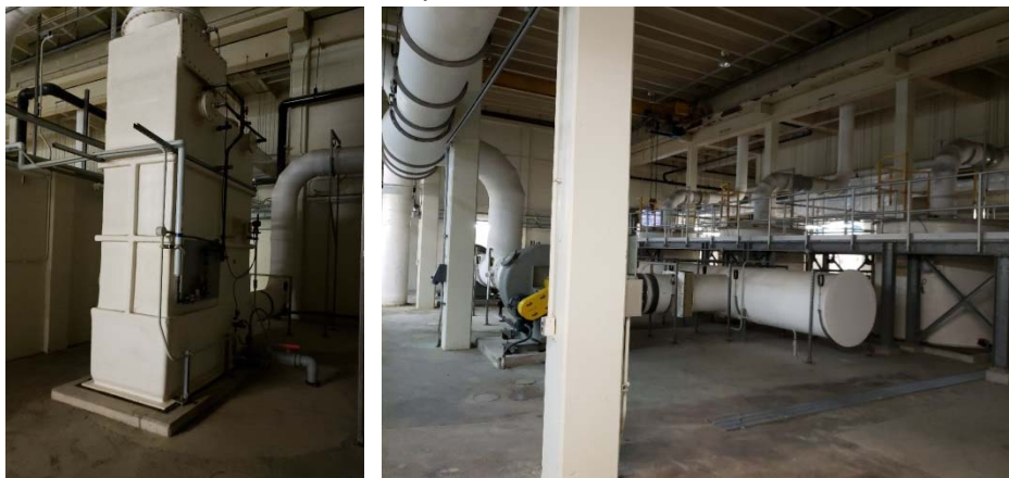
FIGURE 8: ODOR SCRUBBER SYSTEMS (WET SCRUBBER LEFT, CARBON ADSORBERS RIGHT)
