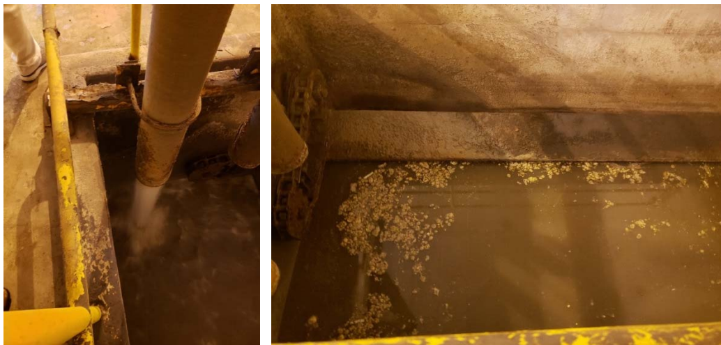
FIGURE 4: TEACUP EFFLUENT DISCHARGE ROOM
