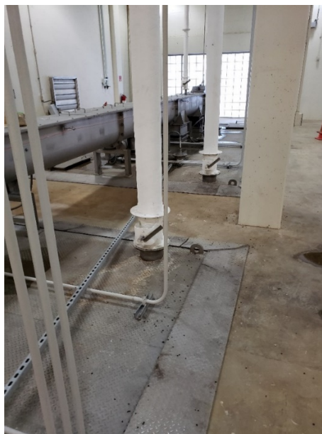
Figure 6-5. Dampers on top of the existing biosolids cake bins
