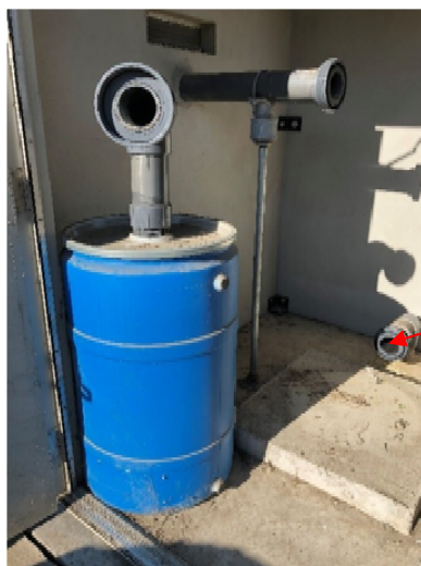
FIGURE 21: CARBON VENT FILTER INLET PIPE
