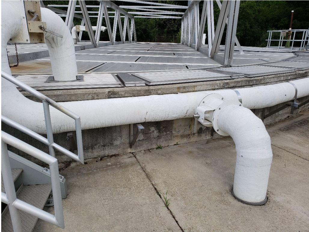
Figure 6-4. Dampers on the existing odorous air duct from the sludge tank systems
