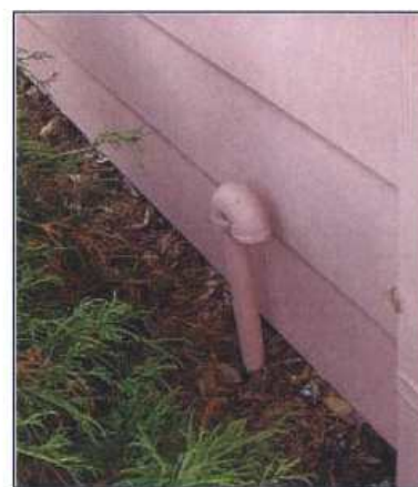
A vent for an underground storage tank is an indication that the tank is still present.
