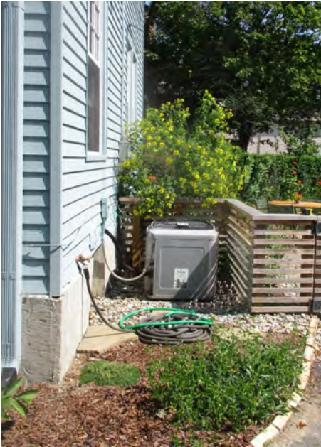
A/C UNIT TO BE RELOCATED
