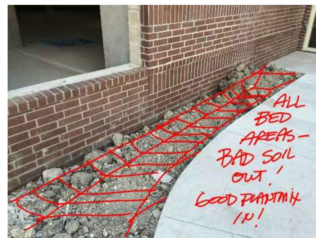
STANDARD - EXCAVATE COMPACTED CONSTRUCTION SOIL FROM PLANTING BED AREAS IN PREPARATION FOR 12" DEEP PLANT MIX IN PLANTING BEDS. FINISH GRADE TO BE AS SHOWN ON CIVIL PLANS
