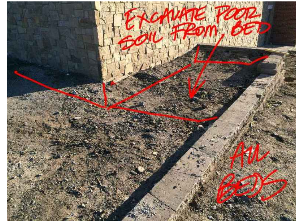
STANDARD - EXCAVATE COMPACTED CONSTRUCTION SOIL FROM PLANTING BED AREAS, TO DEPTH STATED ON PLANTING DETAILS, IN PREPARATION FOR PLANT MIX INSTALLATION.
