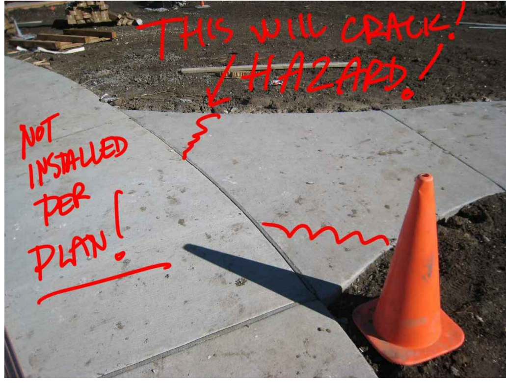
NOT STANDARD - CONCRETE WALKS WITH INCORRECT JOINTING THAT WILL CRACK, AND CAUSE A TRIP HAZARD FOR RESIDENTS AND VISITORS
