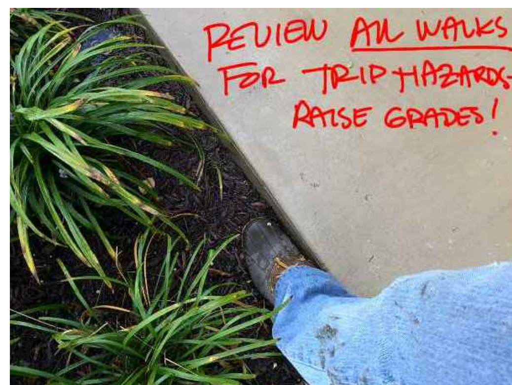
NOT STANDARD - FINISH GRADE TO BE FLUSH WITH EDGE OF WALKS AT LAWN AND PLANTING BED AREAS, TO AVOID TRIP HAZARD FOR RESIDENTS AND VISITORS
