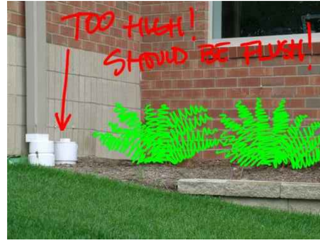
NOT STANDARD - DOWNSPOUT BOOT TOO HIGH, SHOWING ABOVE GRADE
