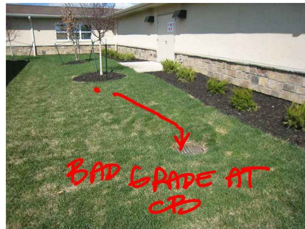
NOT STANDARD / NOT ACCEPTABLE - FLAT GRADE IN LAWN AREA, THEN DROPPING ABRUPTLY AT CATCH BASIN
