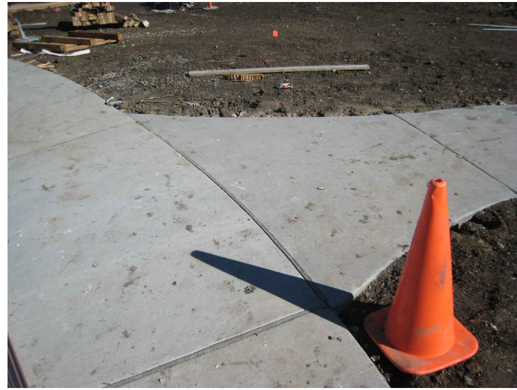
NOT STANDARD - INCORRECT JOINTING ON CONCRETE WALKS
