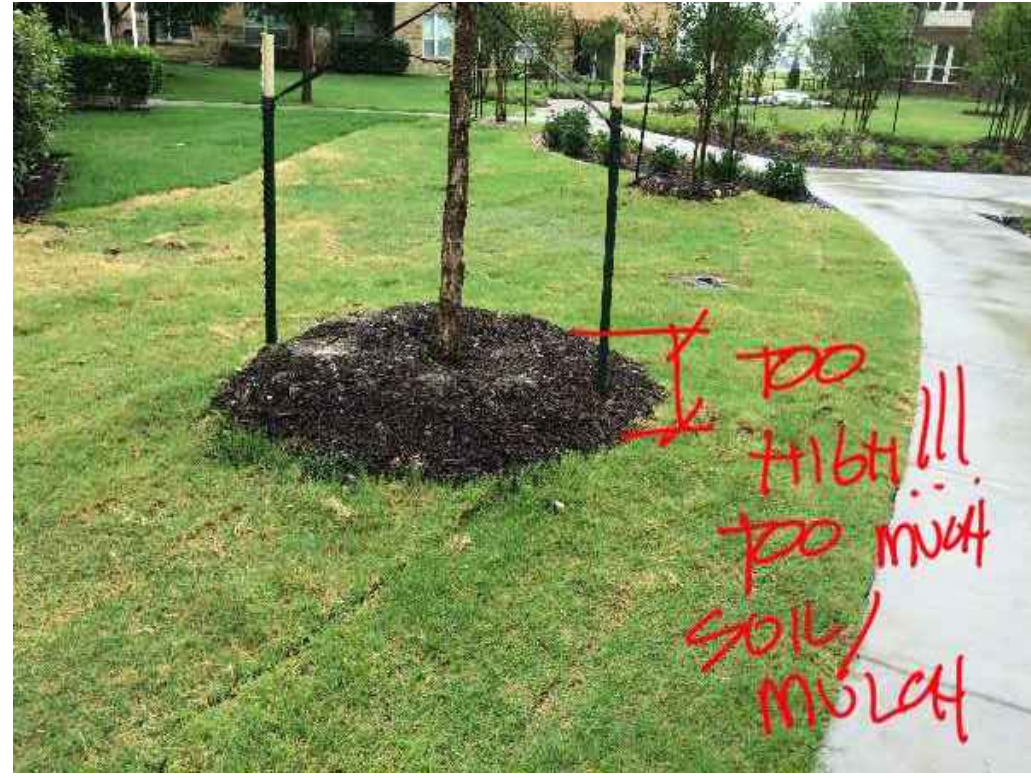
NOT STANDARD - NO MULCH VOLCANOES!!! - THIS CREATES ROT ON THE TRUNK AND KILLS THE TREE. INSTALL TREE PER DETAILS.
