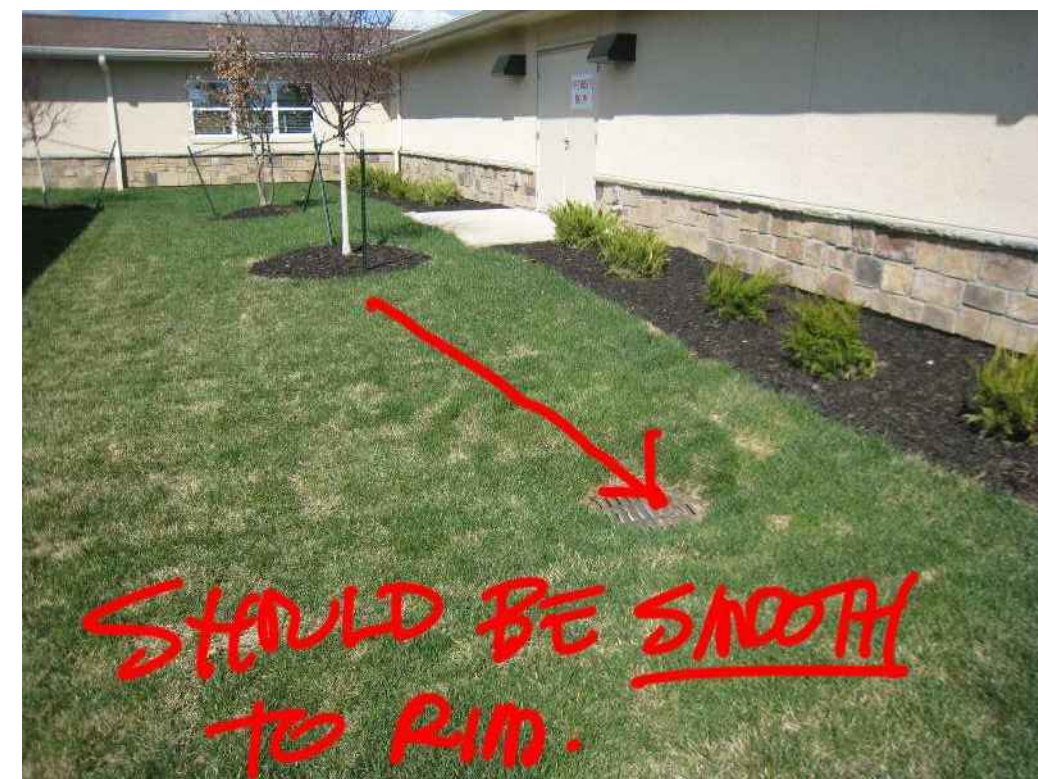
STANDARD - FROM BUILDING OR WALK, PROVIDE A SMOOTH EVEN 2% MINIMUM GRADE TO THE RIM OF THE DRAIN INLET OR CATCH BASIN
