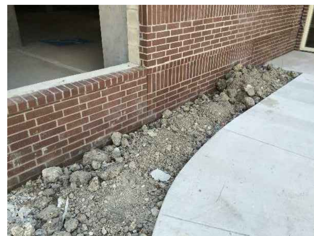
NOT STANDARD - TOO MUCH COMPACTED CONSTRUCTION SOIL IN BEDS.
