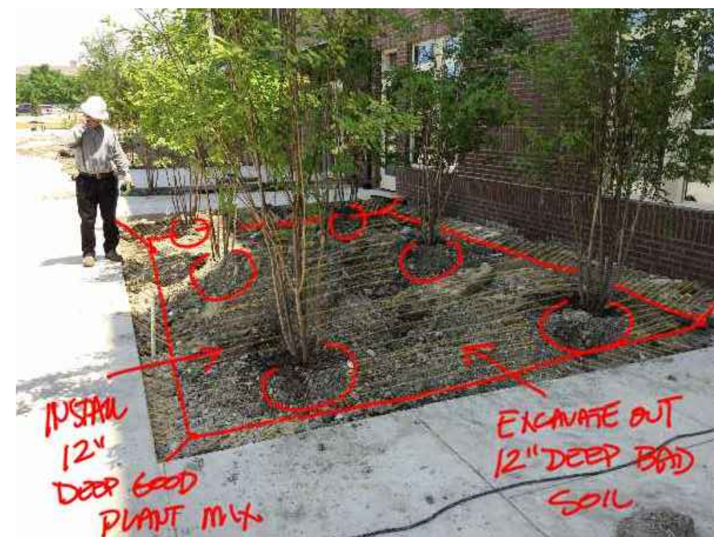
STANDARD - EXCAVATE COMPACTED CONSTRUCTION SOIL FROM PLANTING BED AREAS IN PREPARATION FOR 12" DEEP PLANT MIX IN PLANTING BEDS. FINISH GRADE TO BE AS SHOWN ON CIVIL PLANS
