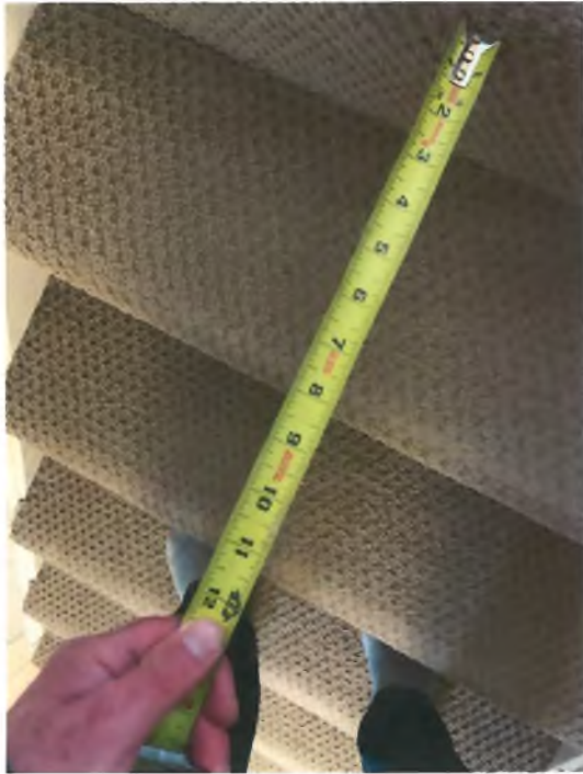
Picture 3: Staircase tread depth is 8"
