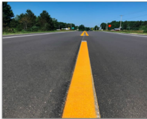
Figure 30 – Recessed Wet Reflective Pavement Markings 5
