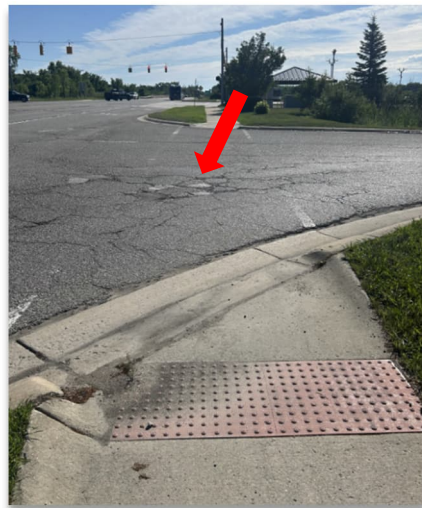
Figure 18 - Faded Crosswalk Marking and Broken Concrete at Southbound US-23 On Ramp
