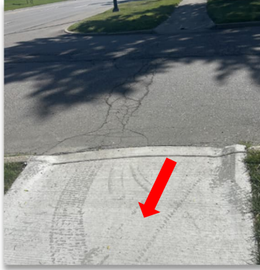
Figure 19 - Missing Detectable Warning Surface at Driveway Crosswalk
