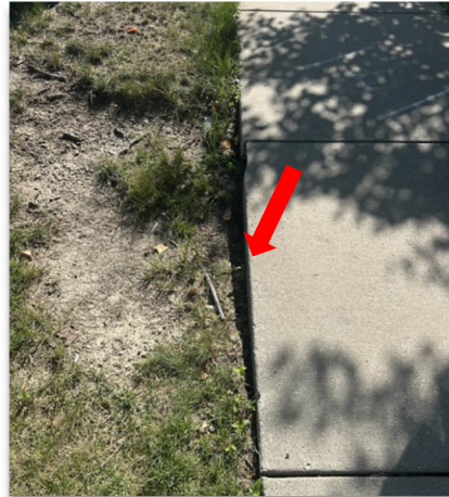
Figure 42 - Depression Adjacent to Sidewalk
