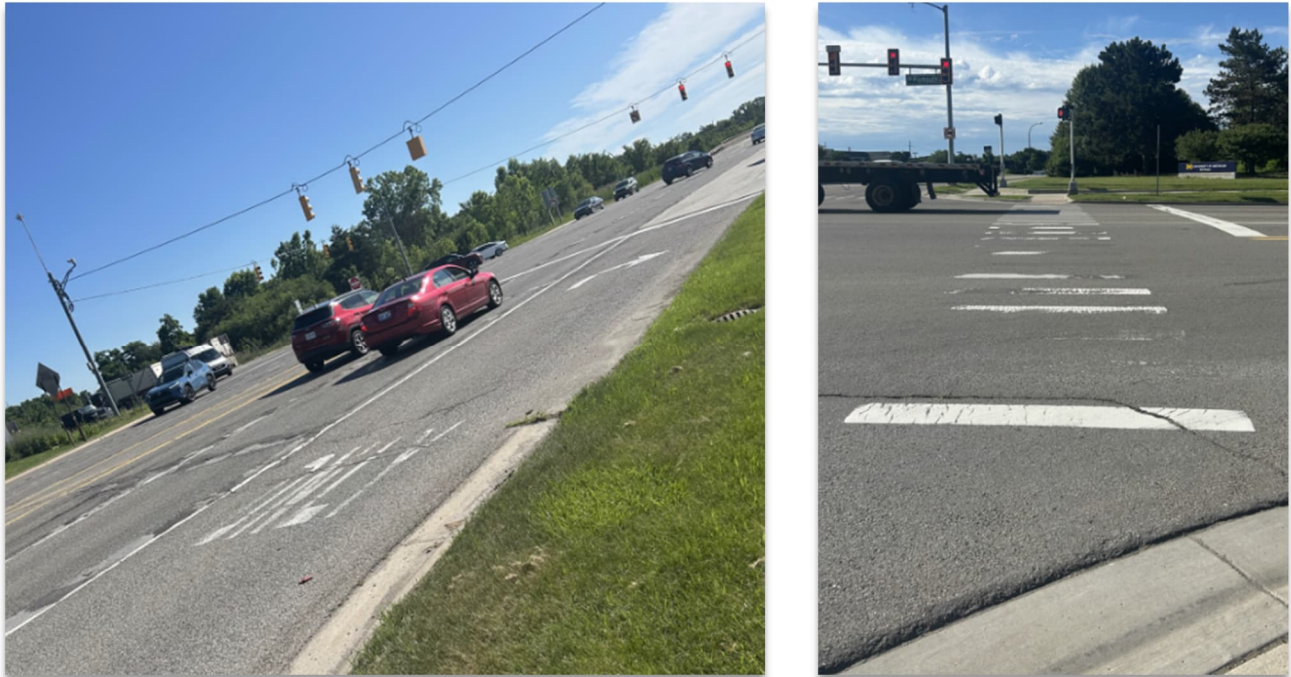
Figure 35 - Faded Pavement Markings
