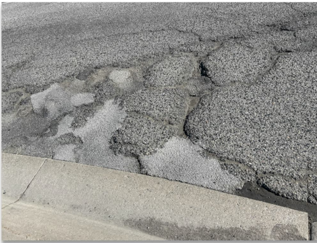
Cracked Pavement on Plymouth Road
