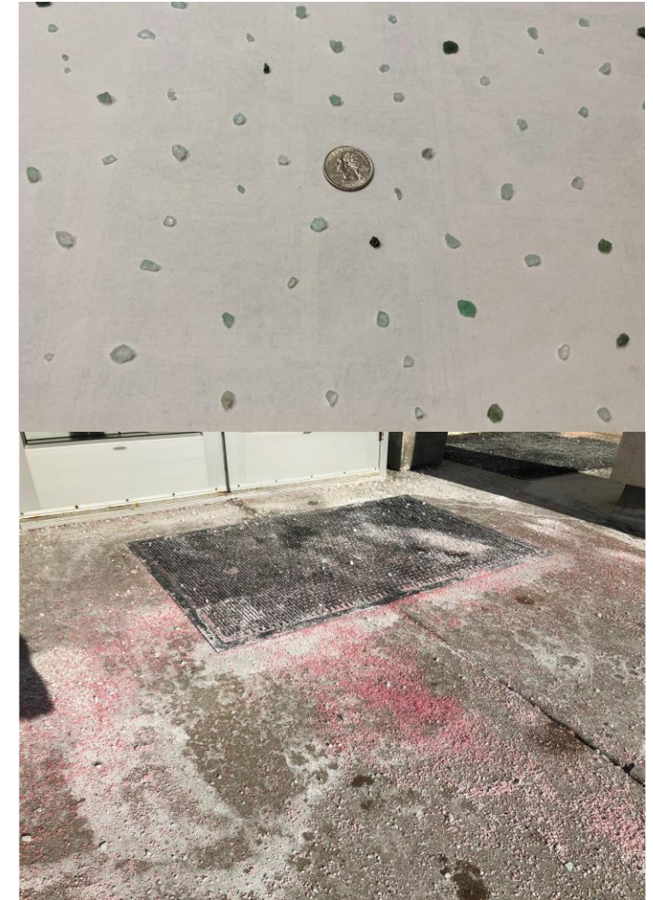
Correct application rate (above) vs incorrect rate (below) for entryways, steps, and ramps. Photos courtesy of U of M
