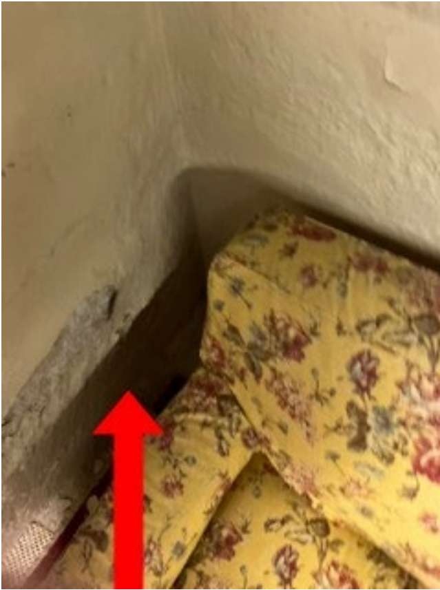
The foundation is flaking/crumbling due to water intrusion
