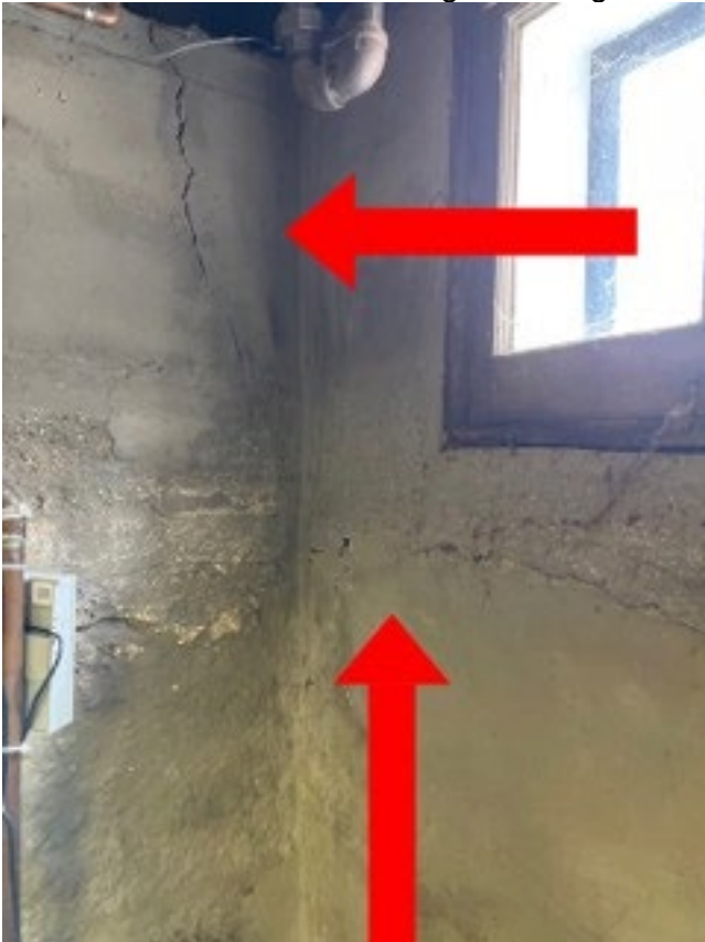
Settling cracks in the foundation, bowing present, the foundation is flaking/crumbling due to water intrusion, active water intrusion in this area
