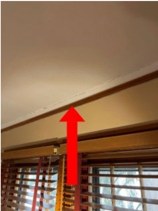
Settling crack in plaster wall covering
