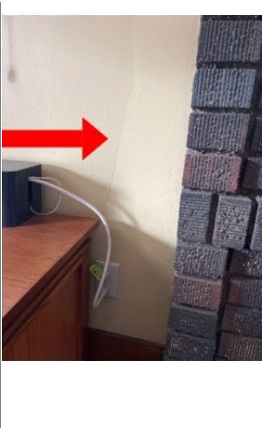
Settling cracks in living room wall
