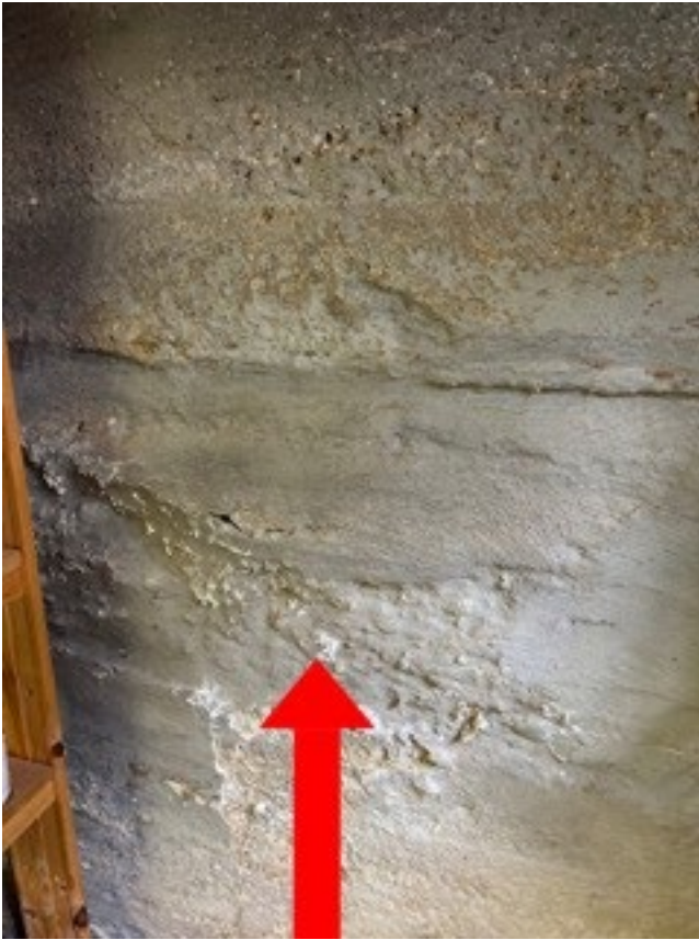
Areas of the foundation are flaking due to water intrusion, horizontal cracking and bowing noted in areas
