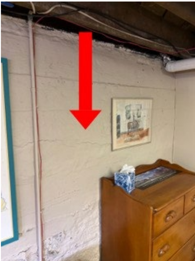
Horizontal cracking/bowing of the foundation, the foundation is flaking due to water intrusion
