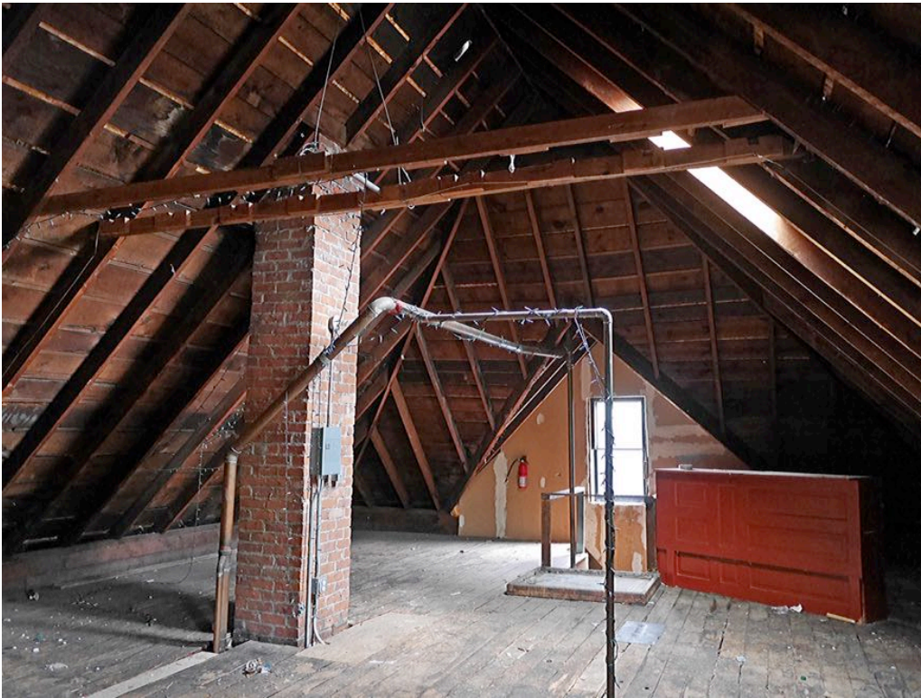
Photo No. 11 (image No. 30): Attic open space looking east. Extra doors were used to create a makeshift bar for parties.
