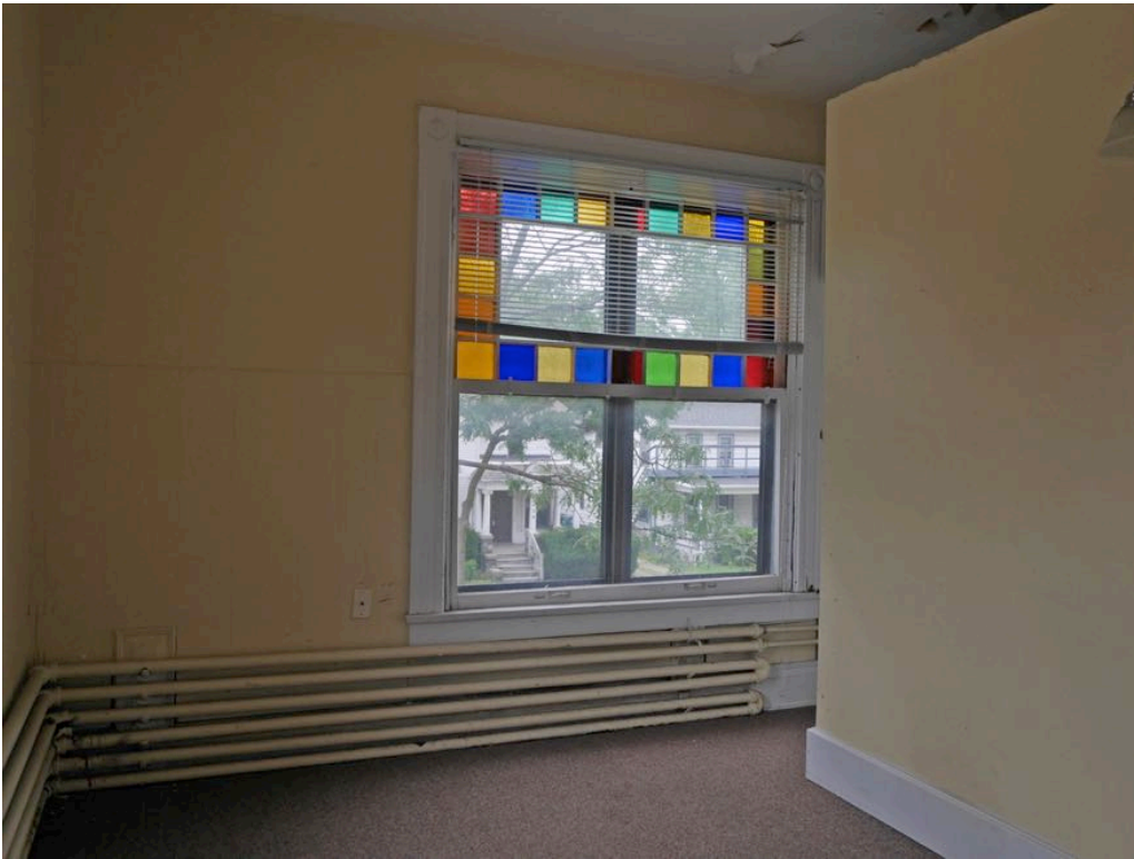
Photo No. 5 (image No. 16): Second floor front bedroom windows have the same colored panes as windows on the first floor. Note unusual radiant heating pipes.
