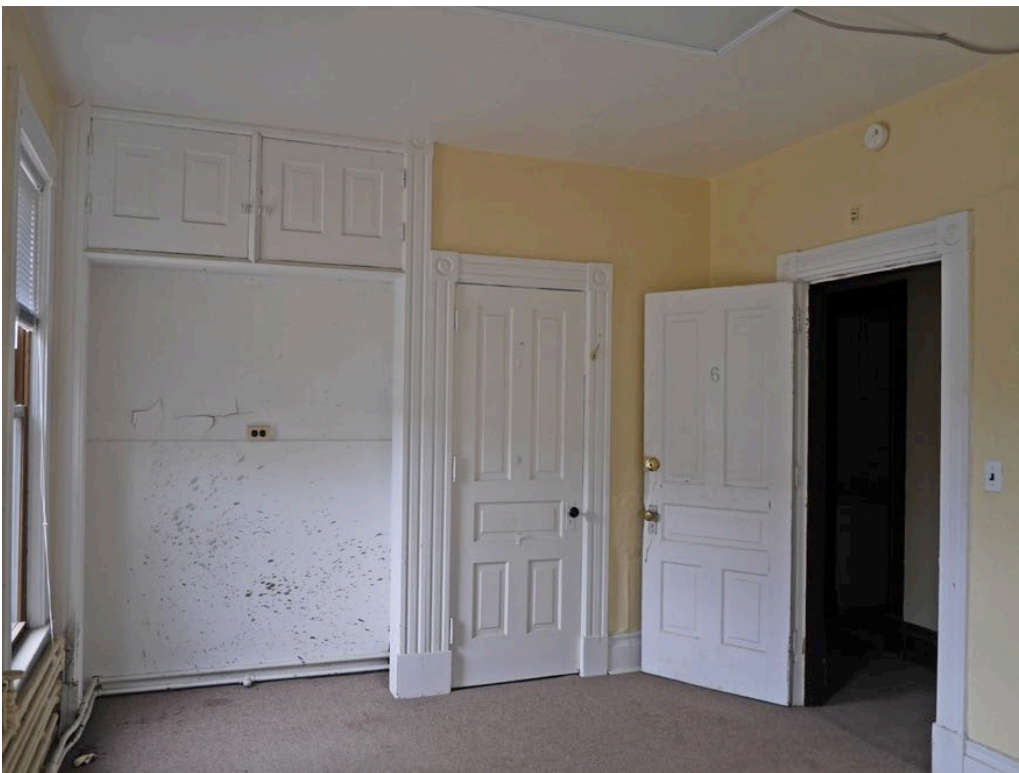
Photo No. 8 (image No. 22): Southeast corner bedroom (BR #6 on second floor sketch plan) with built-in closet and storage cupboards and original doors.
