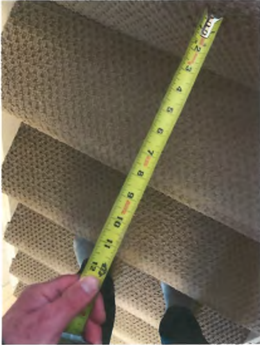
Picture 3: Staircase tread depth is 8"
