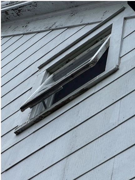
The window has sustained significant water damage
