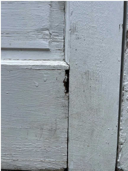
The door has sustained significant water damage
