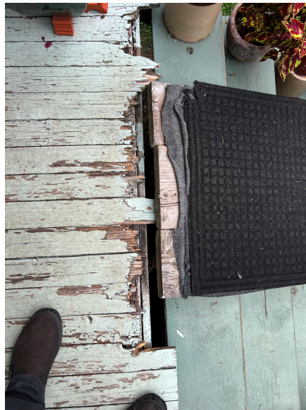
The existing rear porch has significant water damage and deterioration
