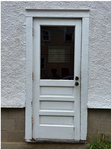
Side door on South Elevation to be replaced
