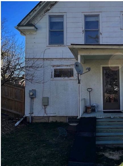
West view of rear elevation; The window to be removed is the awning
