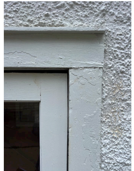
The door does not create a good seal allows air and water infiltration
