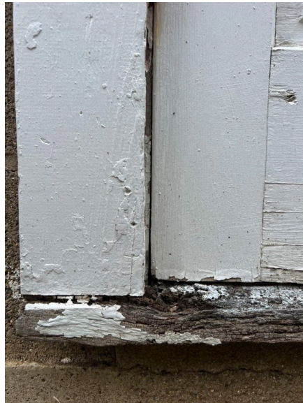
The sill is almost completely deteriorated
