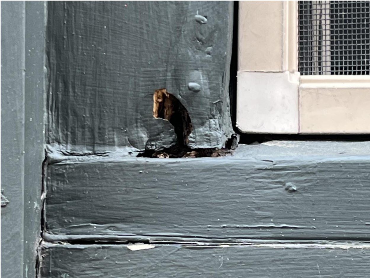
Example of rotting trim:
