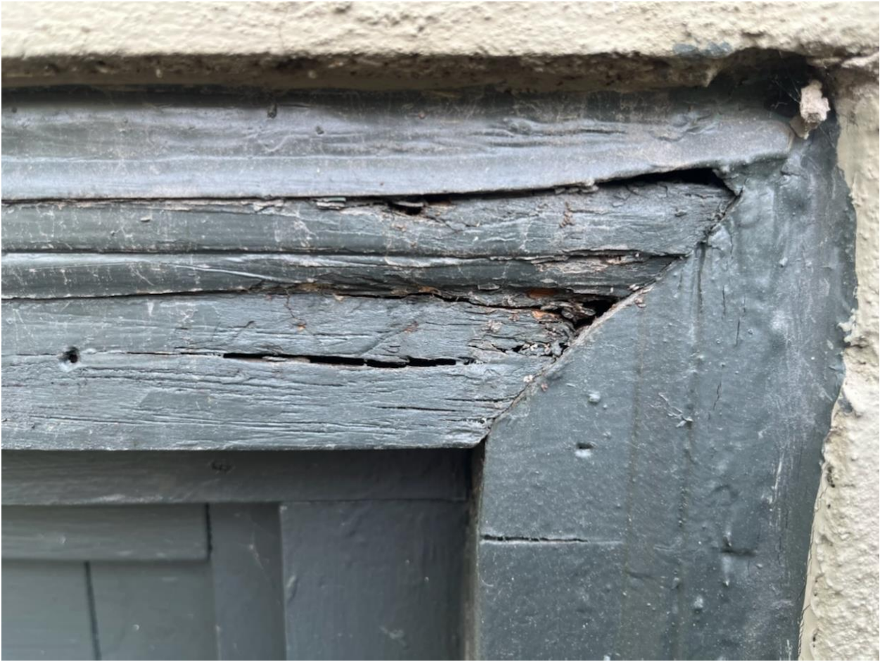
Example of Rotting Trim:
