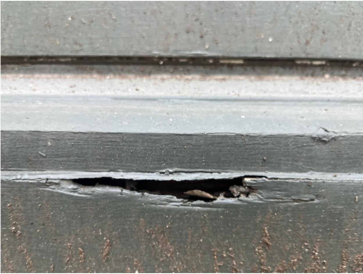
Example of Rotting Trim:
