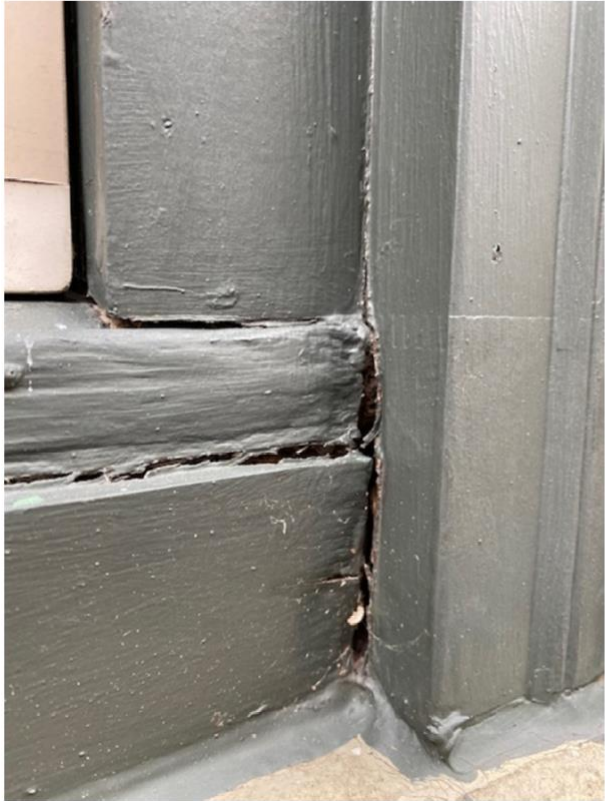
Example of rotting trim and sill with water leakage points:
