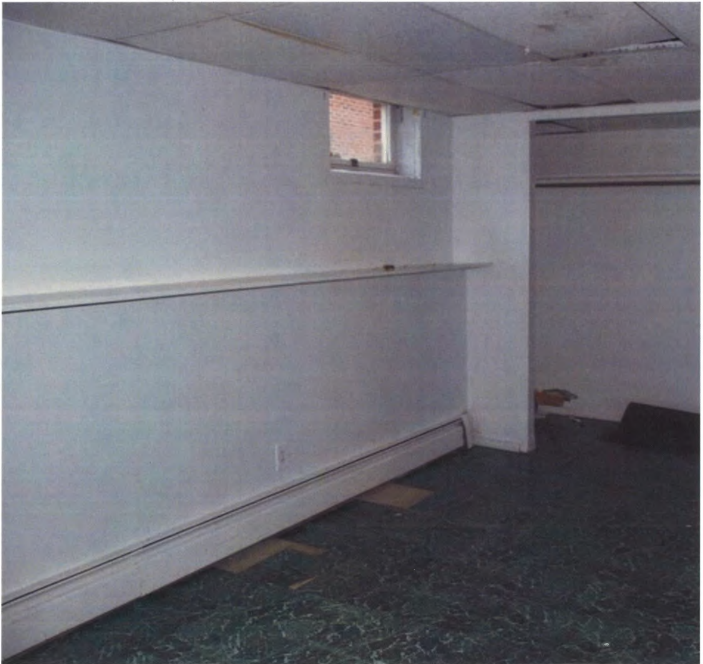
Damaged floors, missing closet door, broken walls and ceiling tiles
