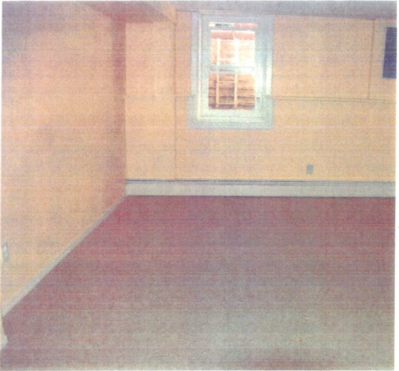
Same room before without furniture. Showing New Egress Window, new electrical box, new flooring, baseboard heating system sanded and painted.
