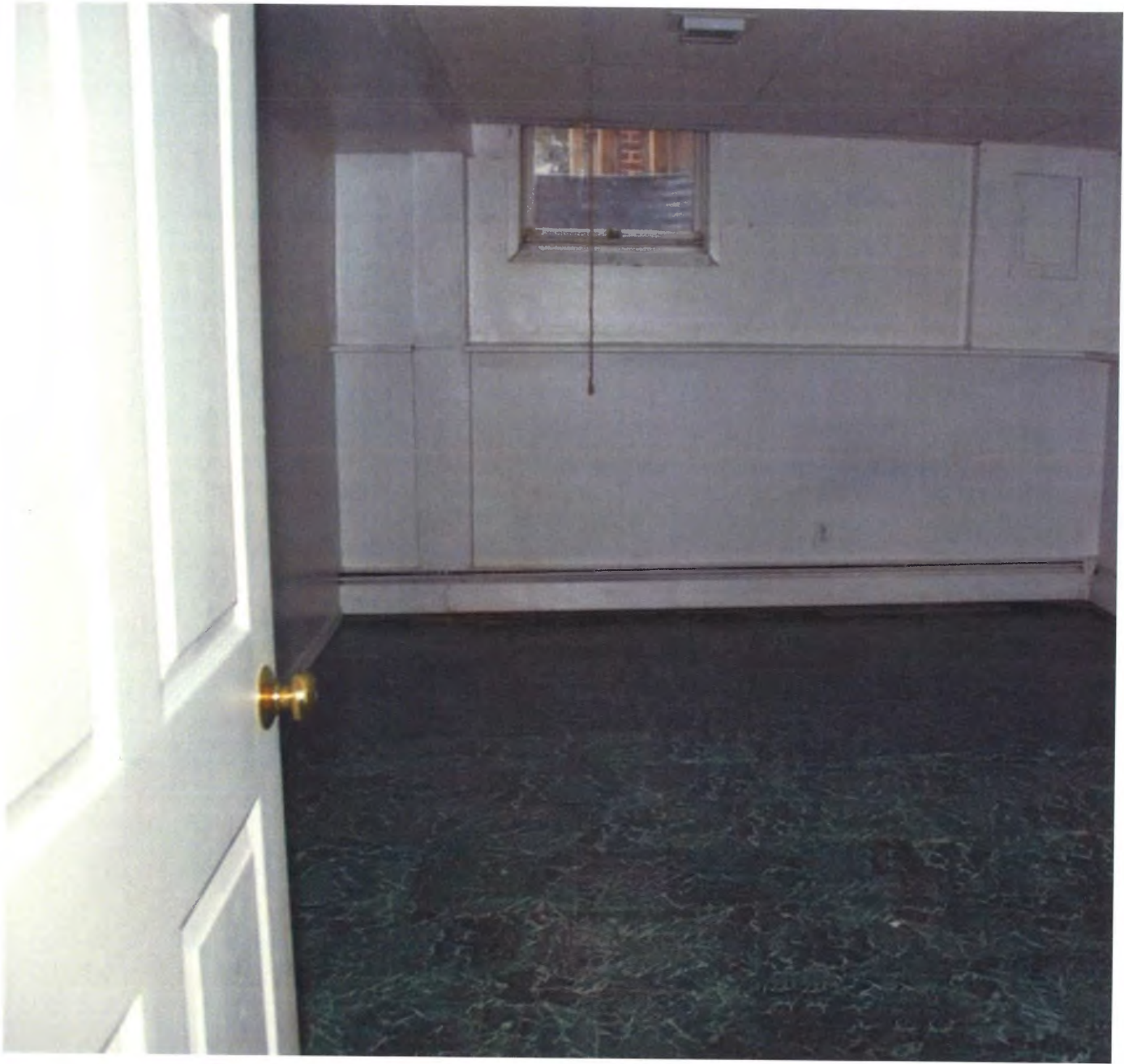
No Egress window, rusted heating baseboard
