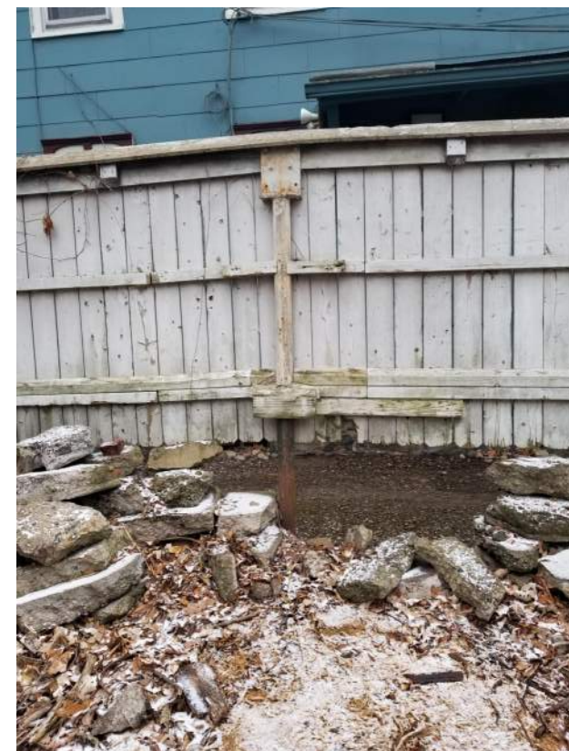
View of failing perimeter fence
