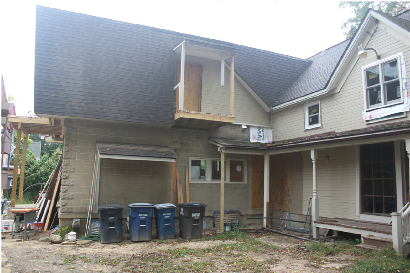
View of Duplex from courtyard showing existing porch roof to be extended
