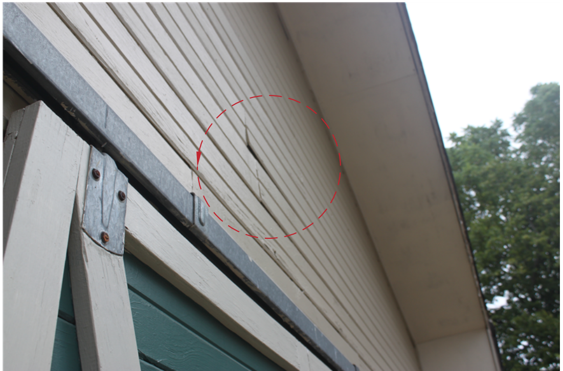
Gaps and cracks typical
