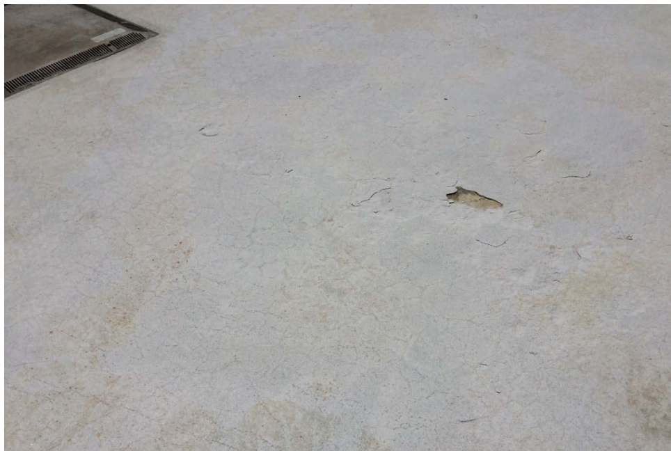
Delaminating Marcite in wading pool
