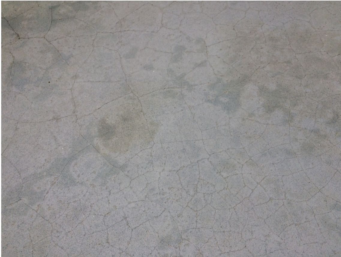
Delaminating Marcite in wading pool
