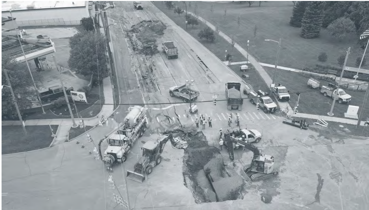
Figure 4-52: June 2021 Water Main Break
