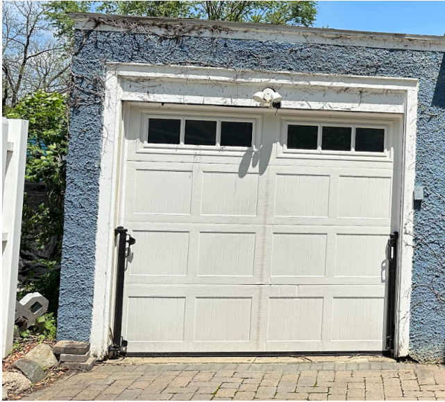
EXISTING GARAGE DOOR IS NOT ORIGINAL
