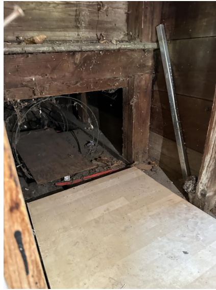
EXISTING BREEZEWAY FRAMED OVER ASPHALT DRIVEWAY (NO PROPER FOOTINGS)
