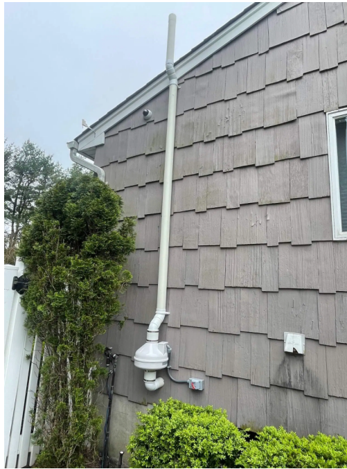
EXAMPLE OF ACTIVE RADON MITIGATION SYSTEM
