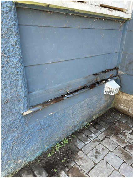
EXISTING BREEZEWAY WALLS WERE BUILT OVER A DECK STRUCTURE AND ARE NOT FLASHED PROPERLY AT THE EXTERIOR
