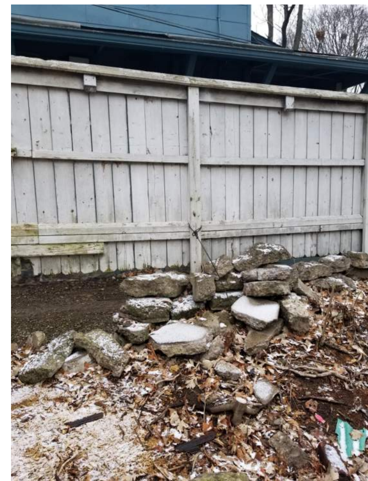
Falling perimeter fence.
