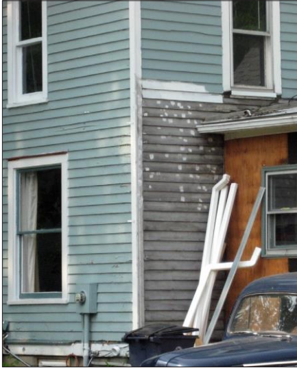
Deteriorated features should be repaired rather than replaced.
