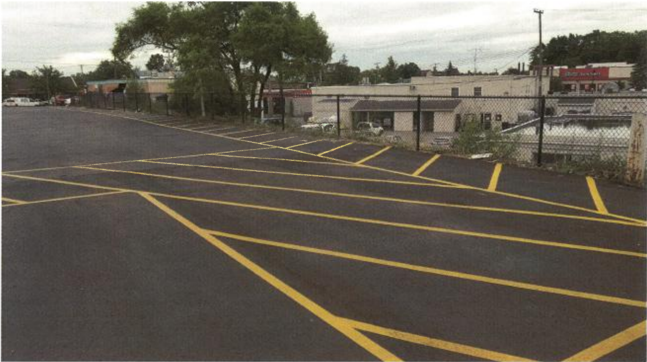
New fencing and pedestrian walkway installed per site plan. Walkway connects to city sidewalk on W Liberty.
