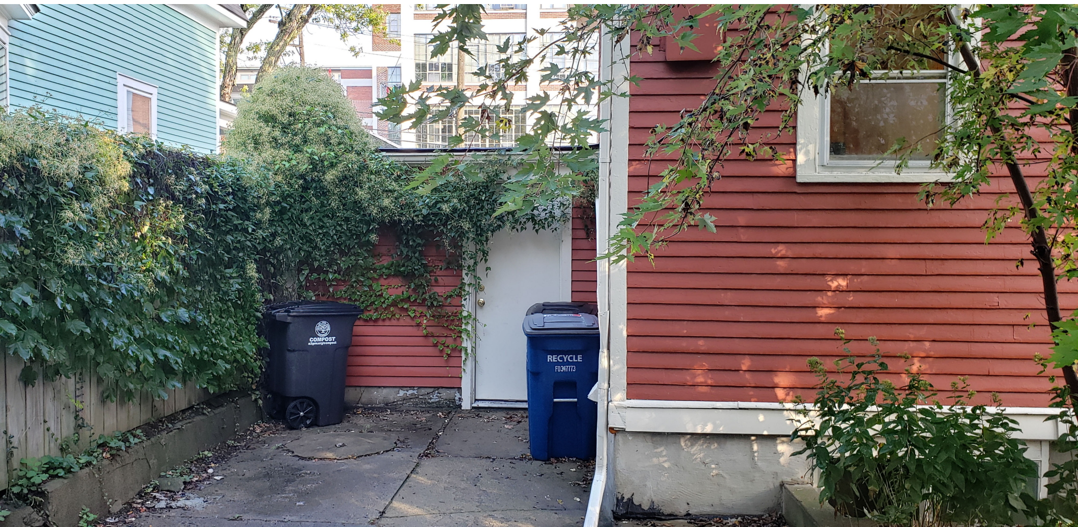
Southwest corner of house looking north: Proposed location of new ADA Restroom
