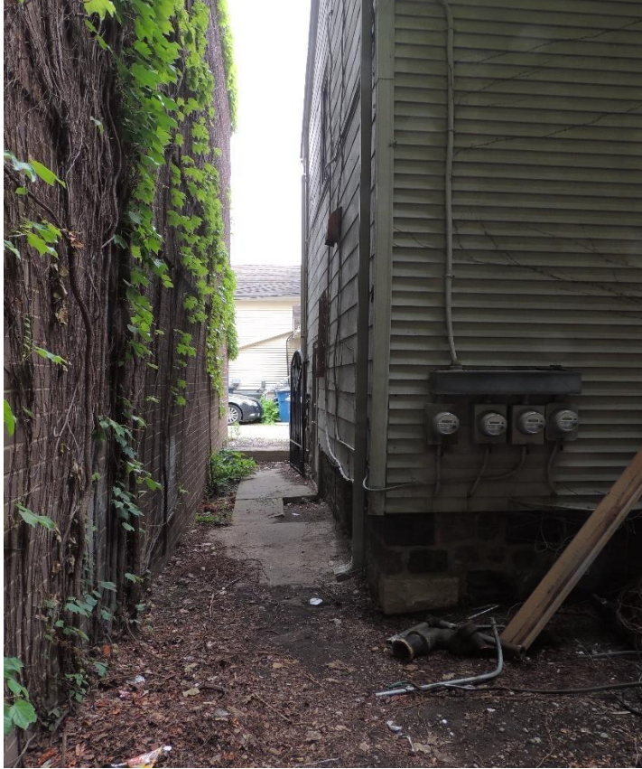
LOOKING OUT FROM THE BACKYARD OF 311 EAST TOWARDS THE BARRIER-FREE RAMP ENTRY POINT SHOWN IN PREVIOUS PHOTO
