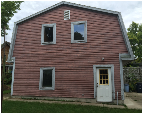
TOP PHOTO OF ORIGINAL 2 STORY HOUSE WITH ADDITION AT REAR WITH DECKS. BOTTOM PHOTO OF ORIGINAL 2 STORY GARAGE SOUTH SIDE.
