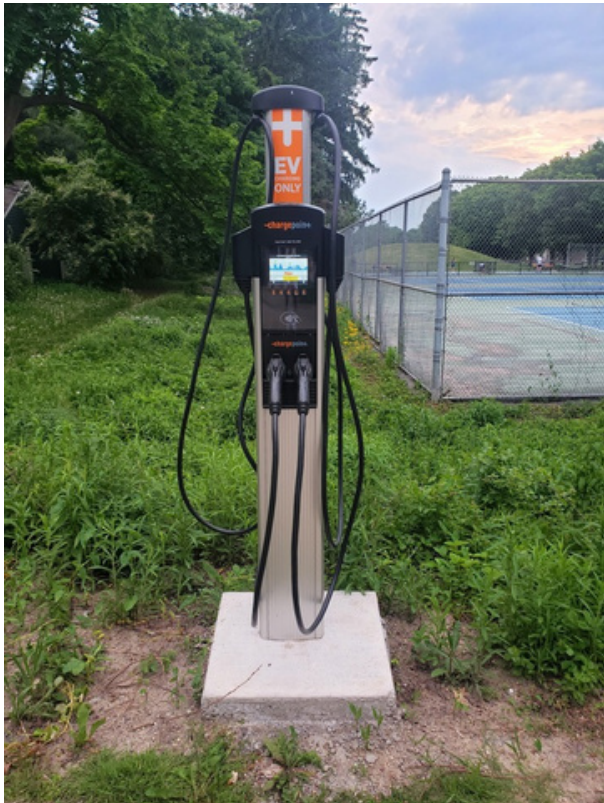
Electric vehicle charging station
