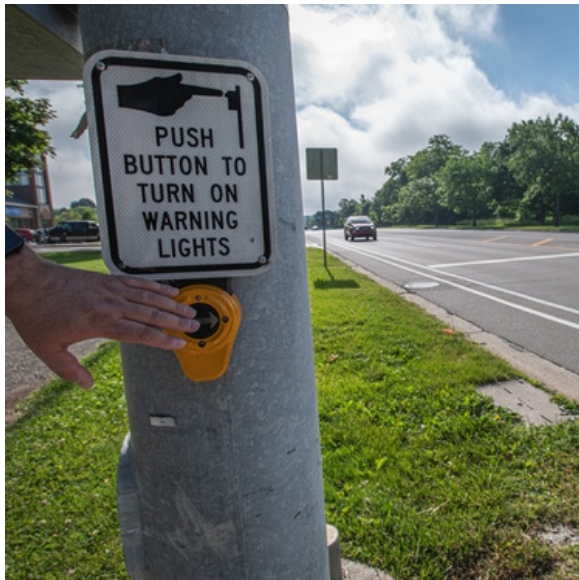
Accessible Pedestrian Signal
