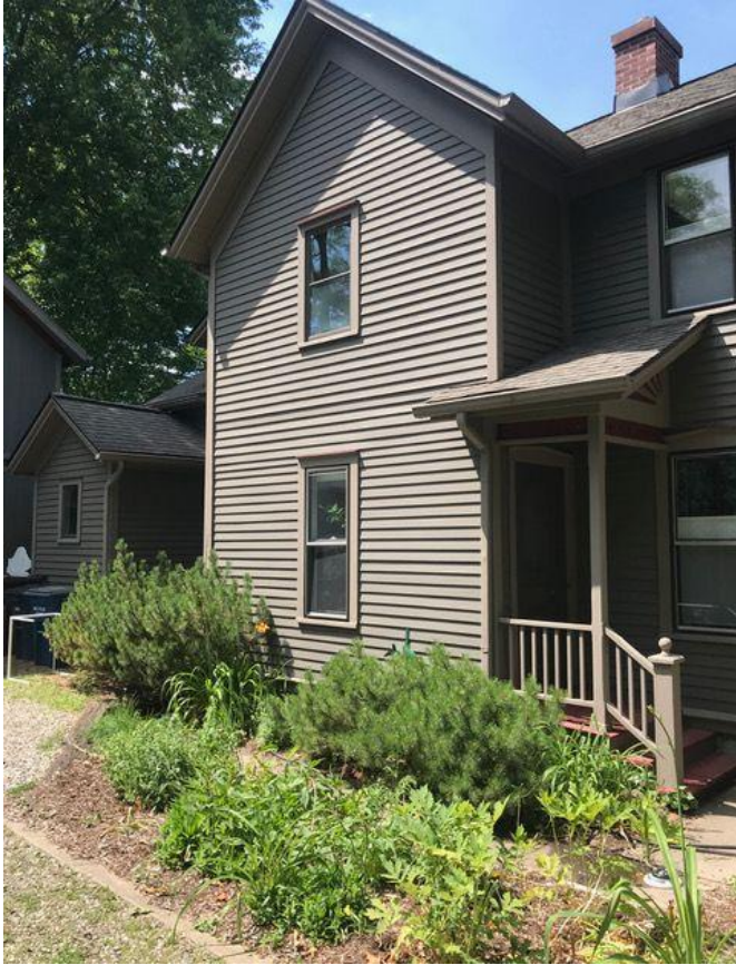
Current south facing view. Second floor window to be updated as egress double hung.
