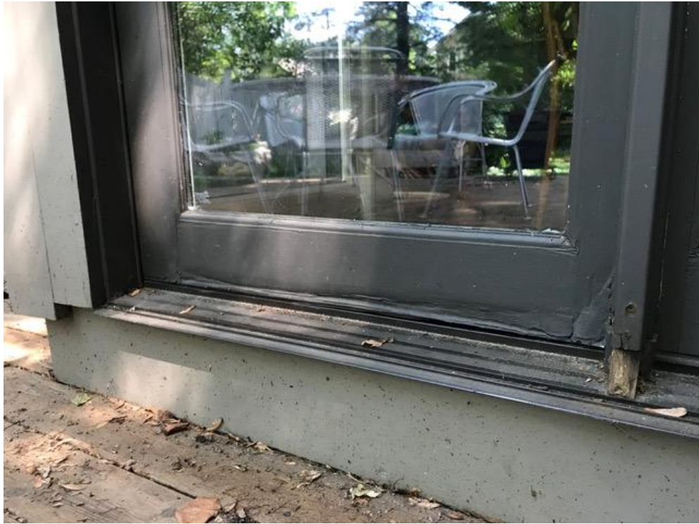
Close up of rotting west facing doors.
