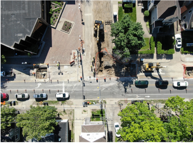
Aerial showing water main isolation valve and water main work at Hoover Avenue and State Street.
