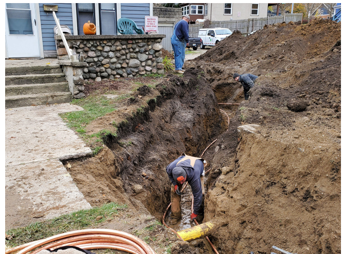
Wade Trim coordinated with the City's Public Works Department to replace lead service lines on Hoover, Greene, and Hill Improvements and suggest a similar approach on State and Hill.
