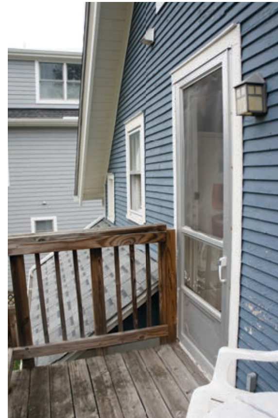
Photo of east elevation upper deck (door to remain-deck to be removed)
