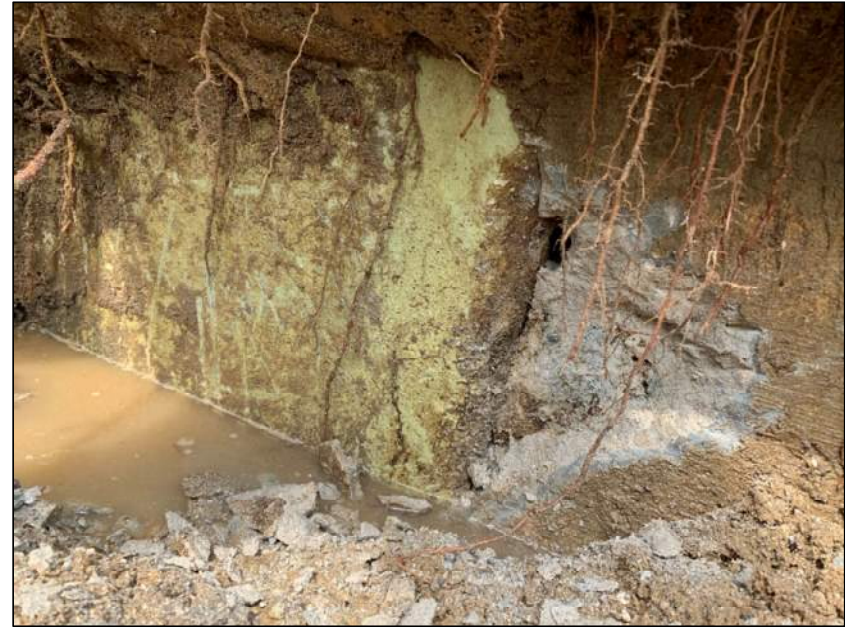
Photo 12: Deteriorated Basement Door Infill Area
