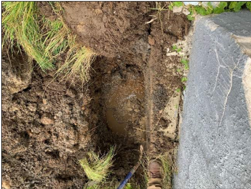
Photo 13: Saturated Soils and Local Erosion along wall and footing
