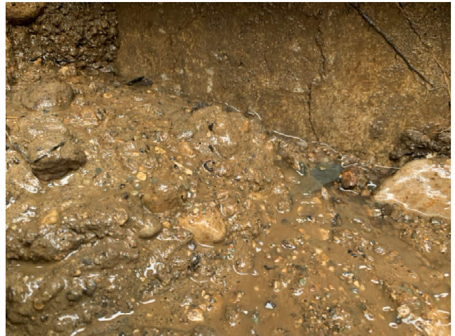
Photo 14: Flowing ground water along East wall
