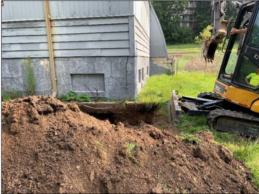
Photo 9: Weeping Corner Wall Cracks
